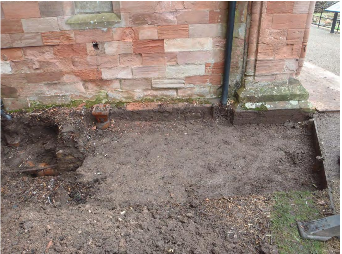
Fig.17 : Completed ground reduction for new path and drainage connection on the west side of the porch
