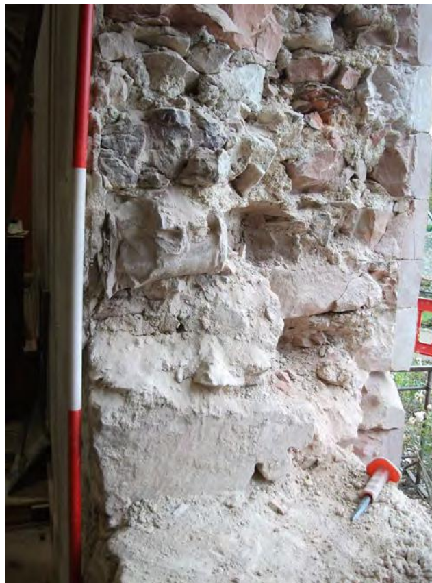
Fig.8 : Detail of west-facing elevation of new door showing architectural fragments in situ
