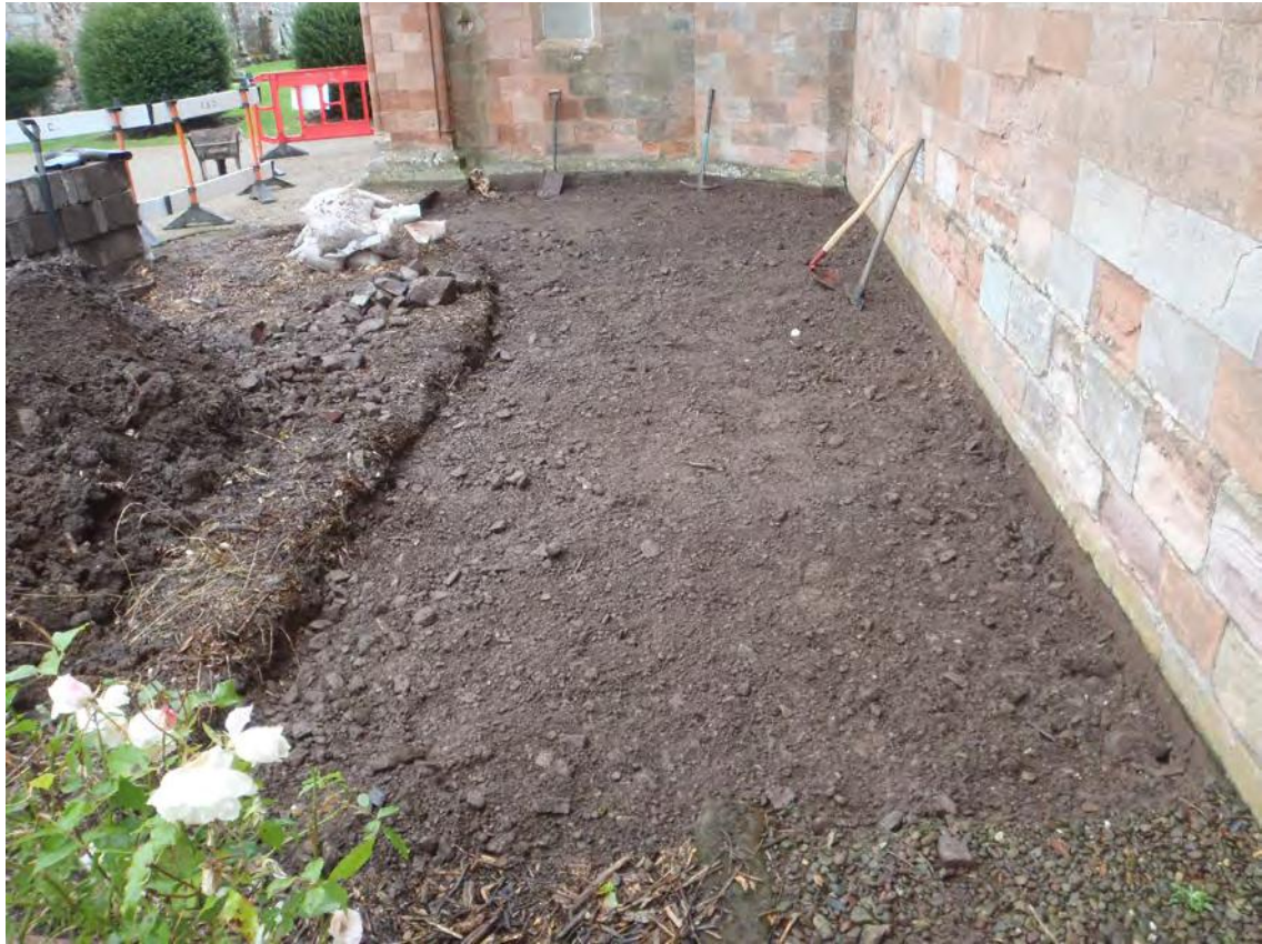
Fig.15 : Completed ground reduction for platt and new path on the east side of porch
