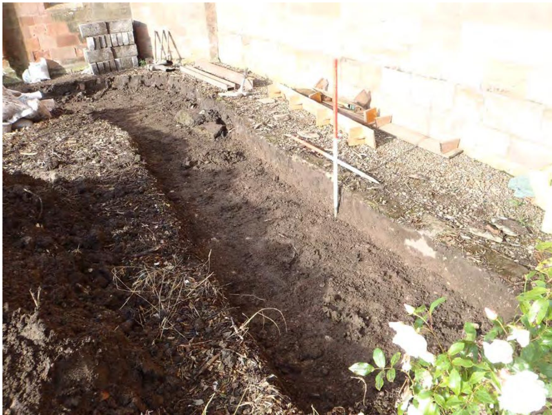
Fig.14 : Excavation in progress for platt and new path on east side of porch, showing kerb stones in situ
