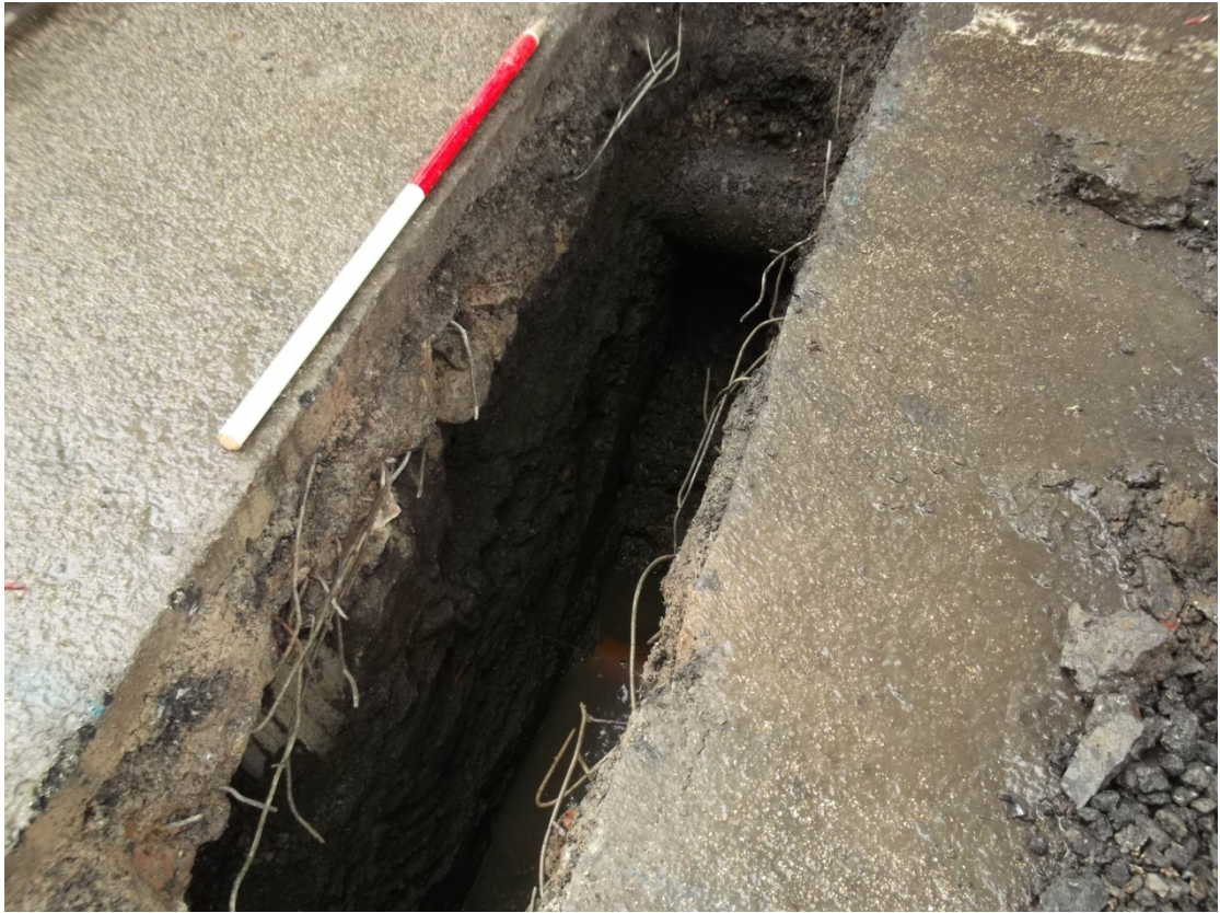
Plate 6: Test Pit 6 extension, oblique shot showing existing pipe work including sewer pipes 124 and 125
