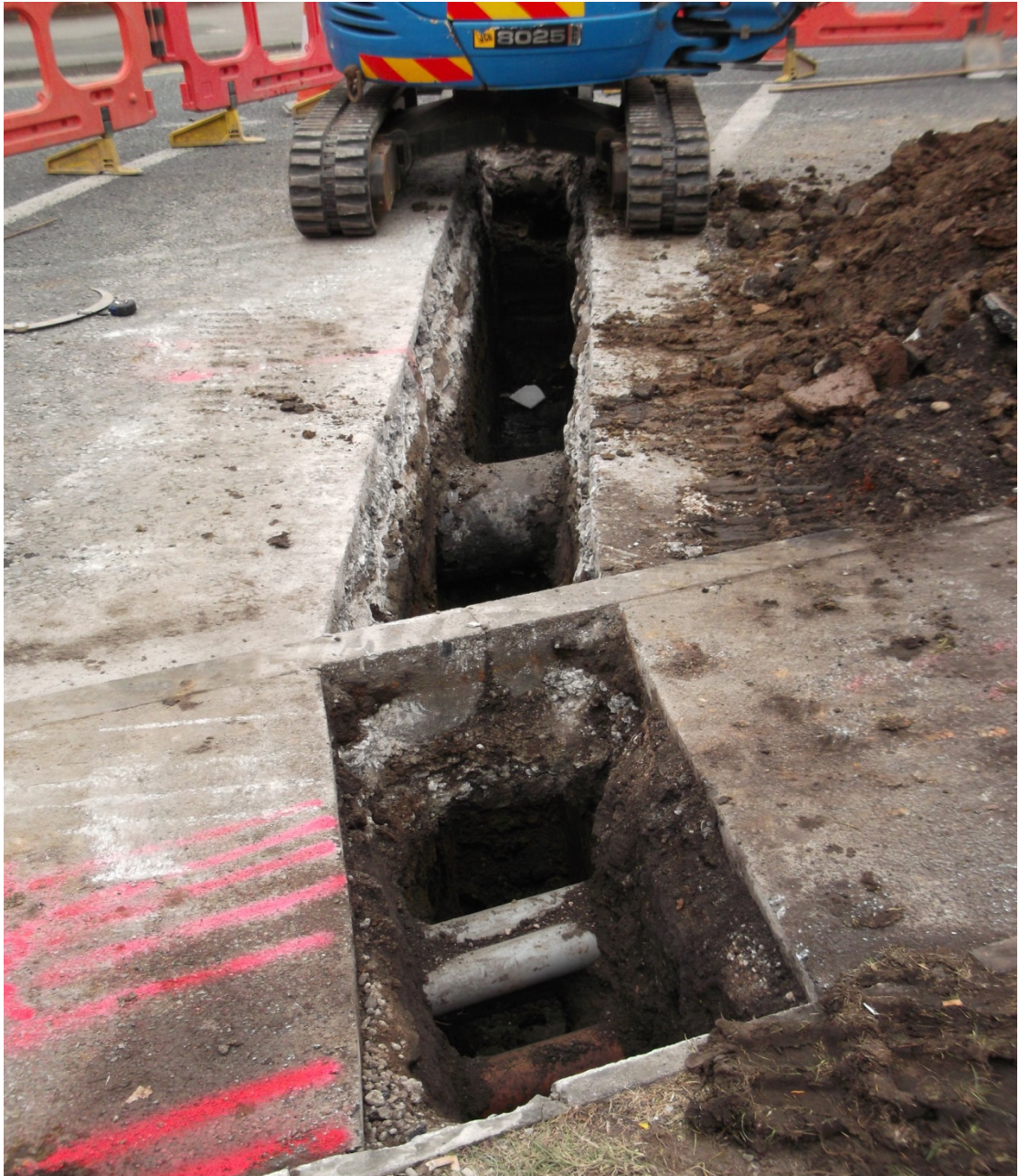
Plate 5: Test Pit 5, oblique plan shot showing existing pipe work including sewer pipe 116
