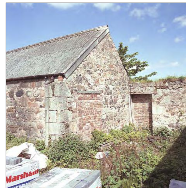
Plate 23 - Range D, East facing gable end and surviving northern wall of demolished East Range.
