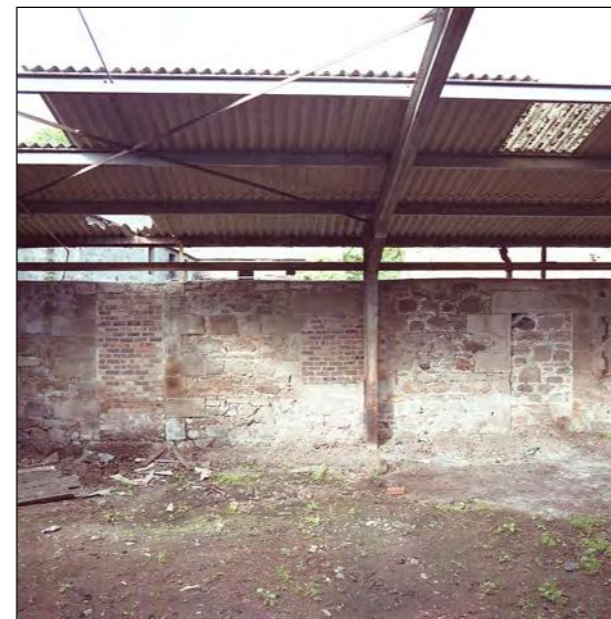
Plate 47 - Wall F. Support wall of the modern cattle court and remaining east wall of the demolished East Range.
