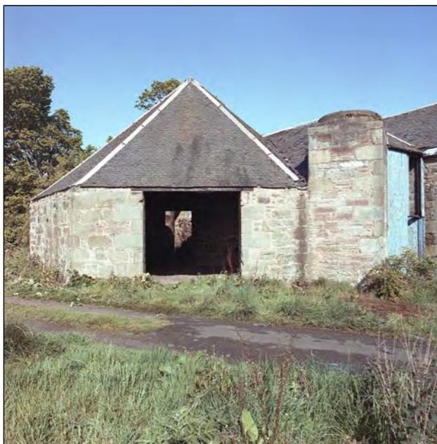
Plate 5 - Range A, South elevation. East side of horse engine house and chimney base.
