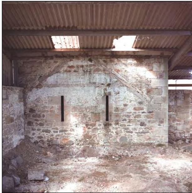
Plate 17 - Range A, East facing gable, showing position of the roof rafter and slit vents.
