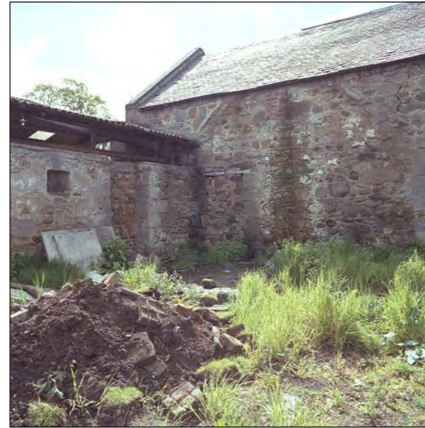
Plate 10 - Range A, North elevation and Wall F junction. The roof raggle above the blocked door can be seen.
