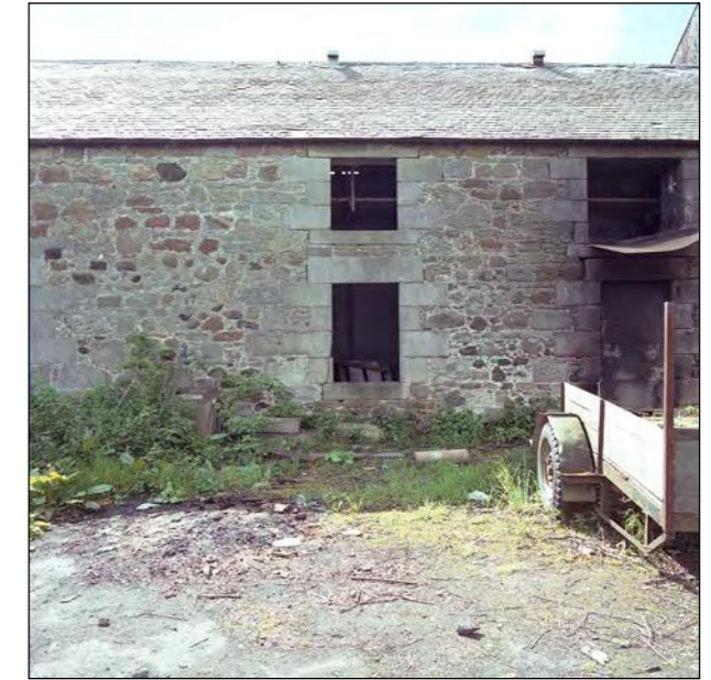
Plate 12 - Range A, North elevation, west end, showing open windows and vents for silos along roof ridge.
