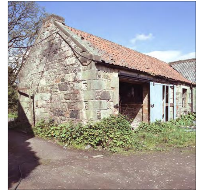
Plate 20 - Range C, South facing gable end and east elevation of tack-room and stable.
