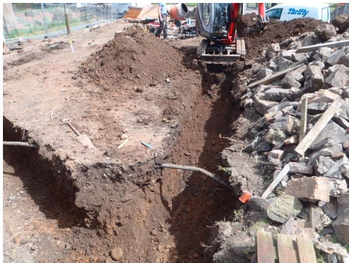
Fig 4. - Working shot showing live service
