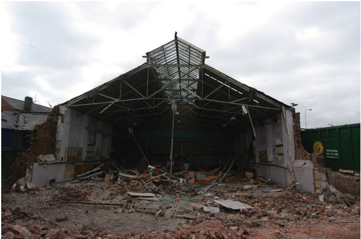
Plate 14 - Building 5 partly demolished showing Prat-type angle-iron roof and clearstory
