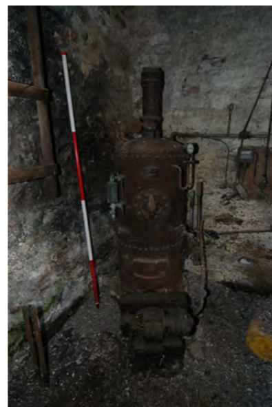
Plate 11: Building 2, Unit 2/4 Boiler room
