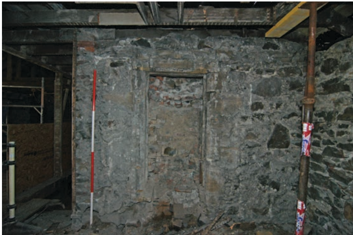
Fig. 27 - Unit 20 blocked window on the early stair tower wall, fabric detail. East-facing elevation
