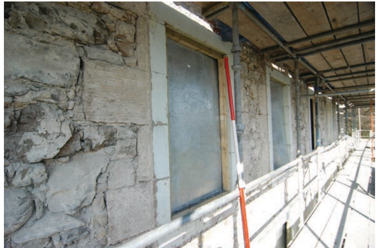
Fig. 36 - Exterior south elevation, dressed stone surrounds around the windows after removal of harling
