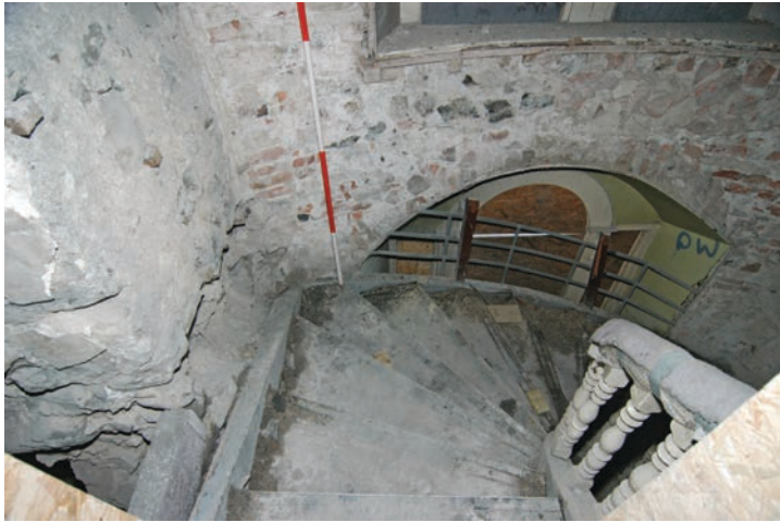
Fig. 33 - Unit 23 abutting later staircase wall and earlier stair tower wall (south-facing elevation)
