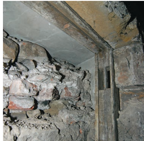
Fig. 28 - Unit 20, blocked window on the early stair tower wall, later wooden window frame
