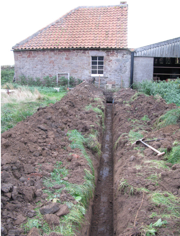
Fig. 2: Cable trench towards buildings
