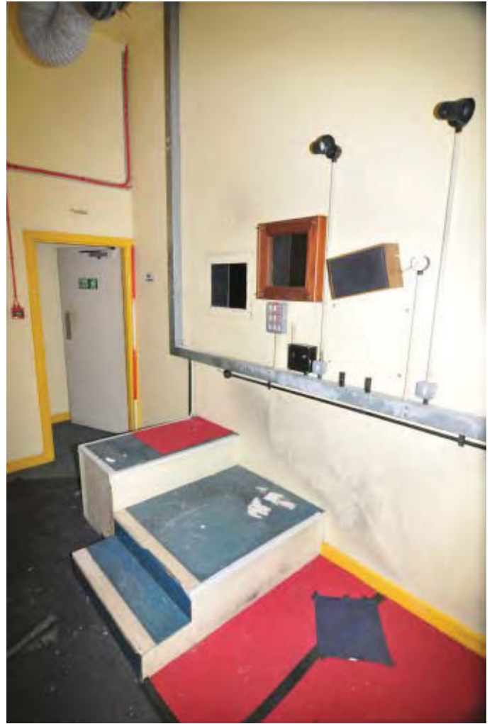
Plate 19. Interior of Cinema 5 projection room
