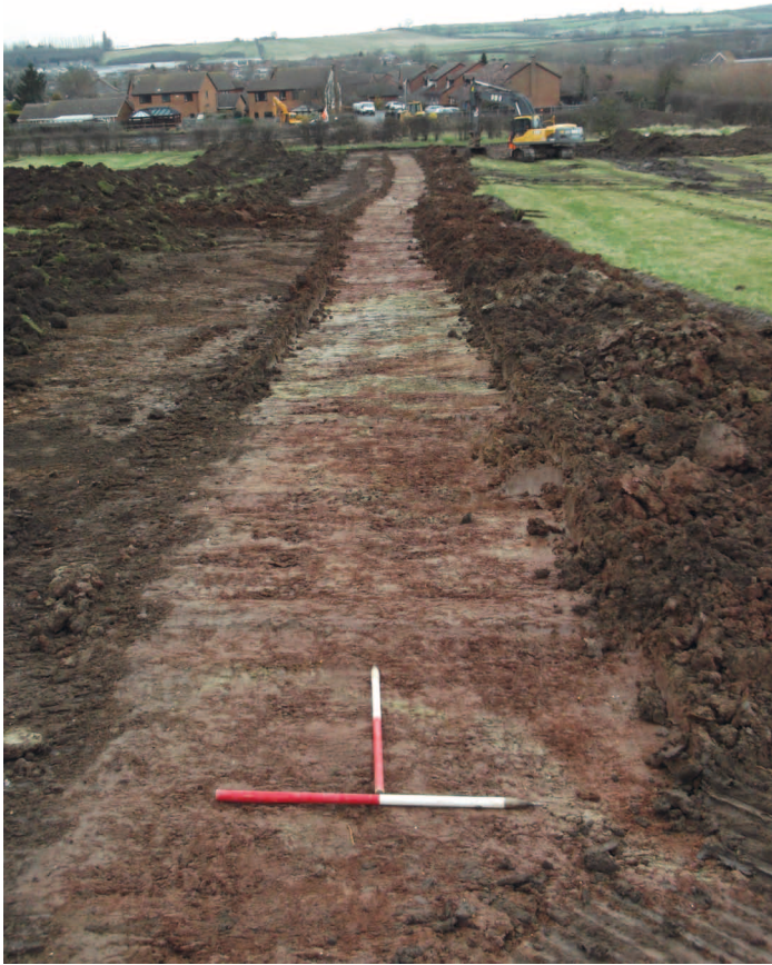
Fig. 3 - North-facing shot of the central spine road from the south of site following excavation
