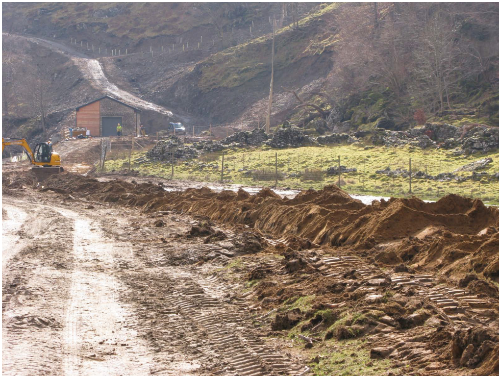
Fig. 3 - Power house access road looking towards the power house from NW - spoil heaps running across the centre of the image indicate the position of the cable trench
