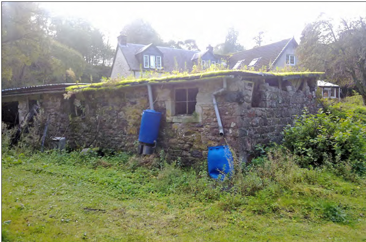
Plate 2 – North and east-facing elevations of the mill with a roof prior to removal
