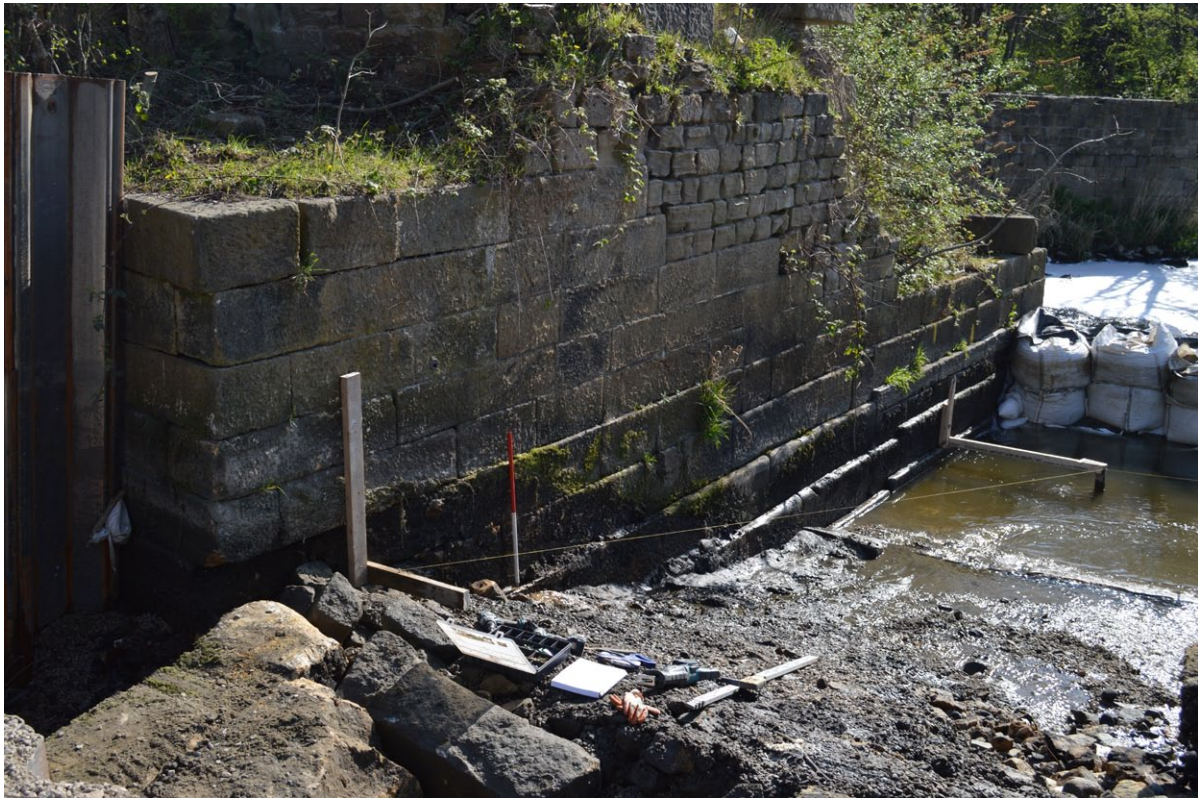
Plate. 3 - North-east-facing shot of St. Ann's Mill Weir following removal of Weir Surface 001
