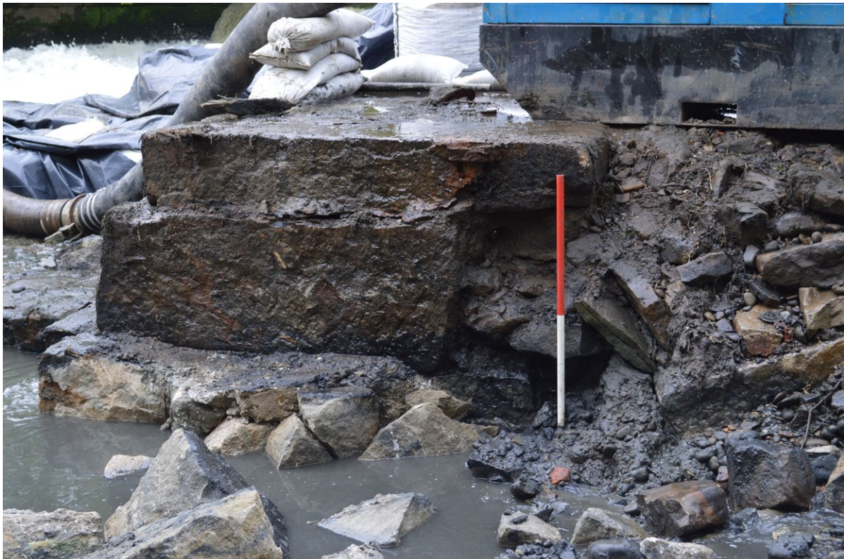
Plate. 8 - East-facing profile of Weir Head 103 and Weir Wall 104 following excavation of the fish pass area
