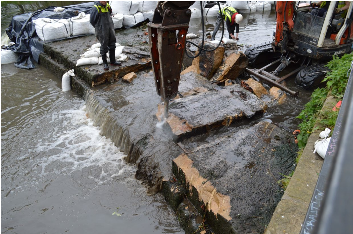
Plate. 6 - Working shot of breaking up of the Weir Head (103) at Burley Mill Weir
