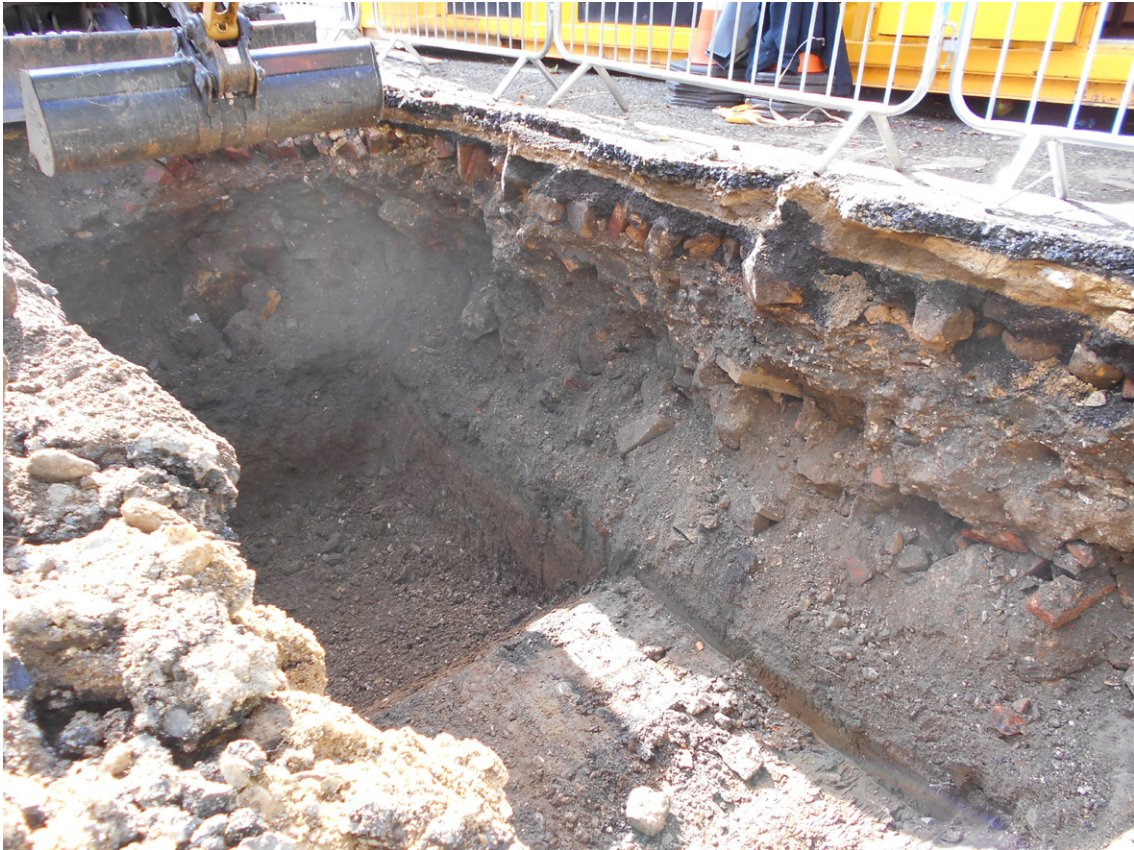
Plate 5 - View of Trench 5, facing south-west, excavated to a max. depth of 2.4m
