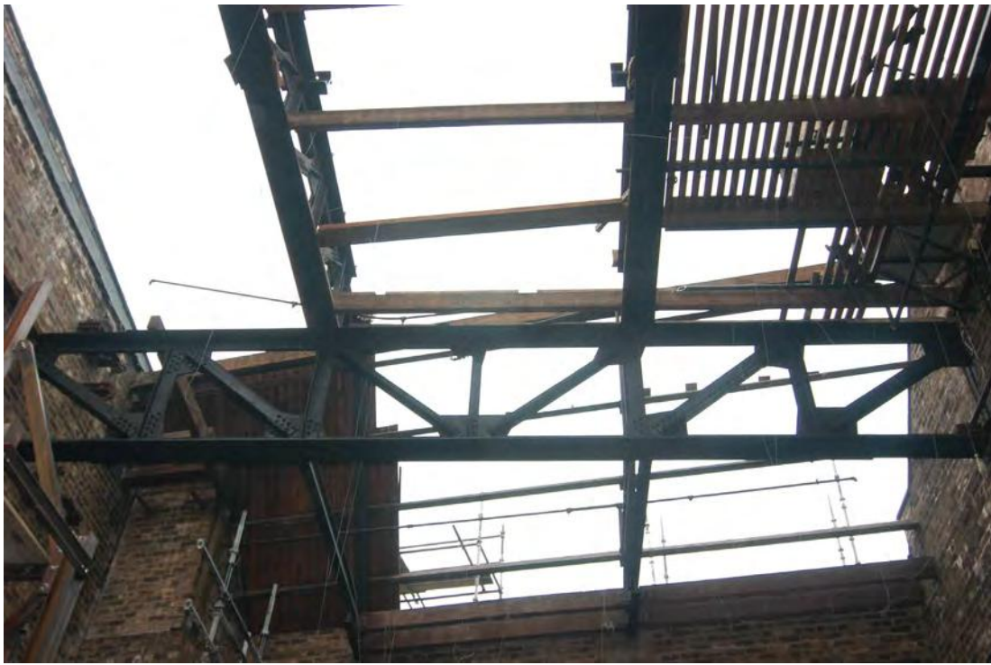
Plate 1: One of two main supporting Pratt trusses showing its rivet and lattice construction (004)
