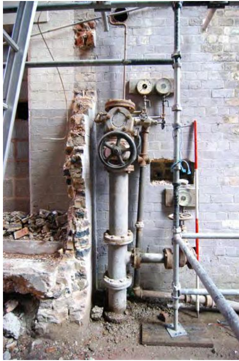
Plate 9: External mains riser and sprinkler shut off valve (051)
