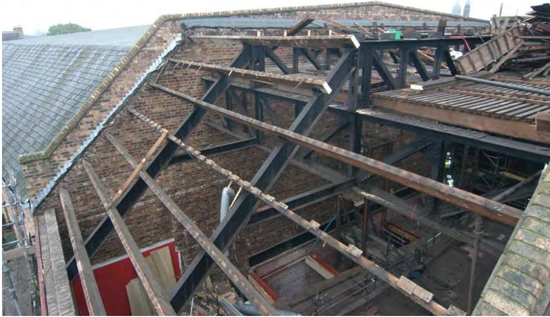
Plate 5: The mansard jack-trusses supporting the timber purlins, the attic floor can also be seen (035)
