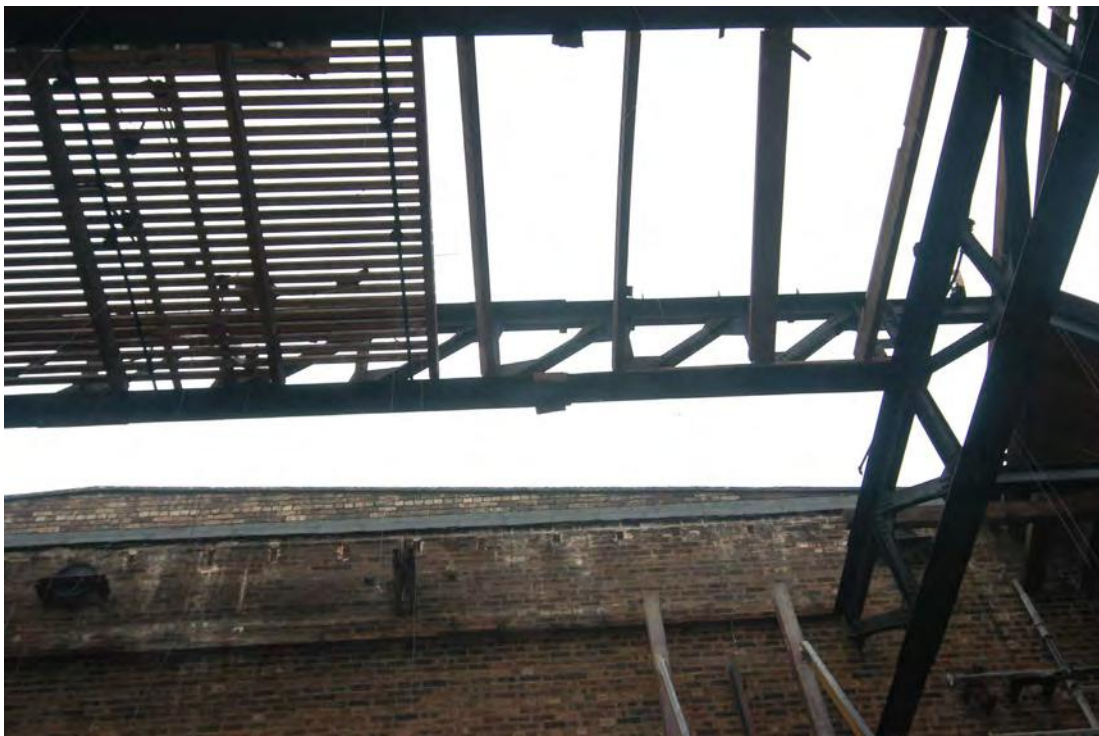
Plate 2: One of two lateral trusses carried on the main Pratt support beams (005)
