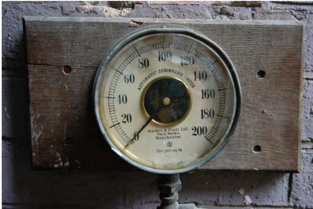
Plate 10: Detailed shot of one of the pressure gauges made by Mather and Platt, Manchester (053)
