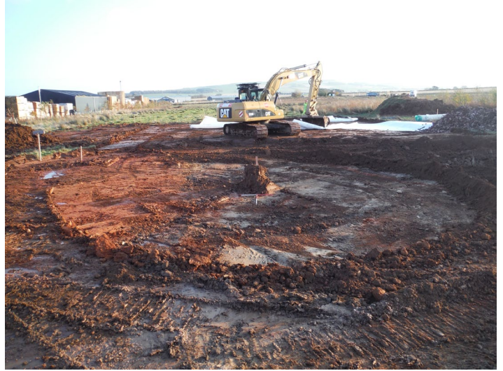
Fig. 3 - 12m diameter turbine base excavated to natural and 20m diameter working area excavated to formation depth.
