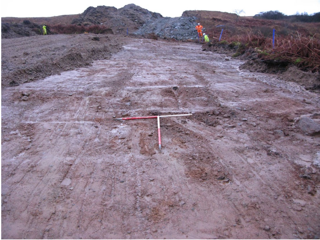
Fig. 4 - Service road stripped to natural (000) and spoil storage area to the south-east
