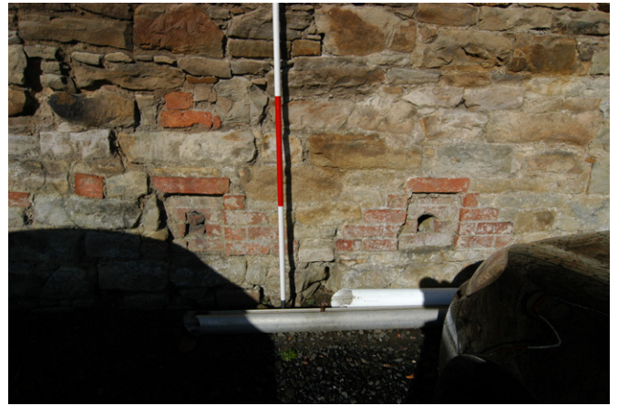
Plate 8 - Interior SE-facing elevation, blocked vents at the base of the wall
