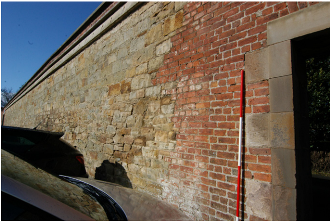
Plate 7 - Interior SE-facing elevation, stone built wall and the roofline of a former conservatory
