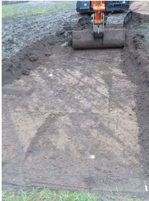
Fig. 3 General shot of the east end of the site after topsoil strip with plough scars, north-facing
