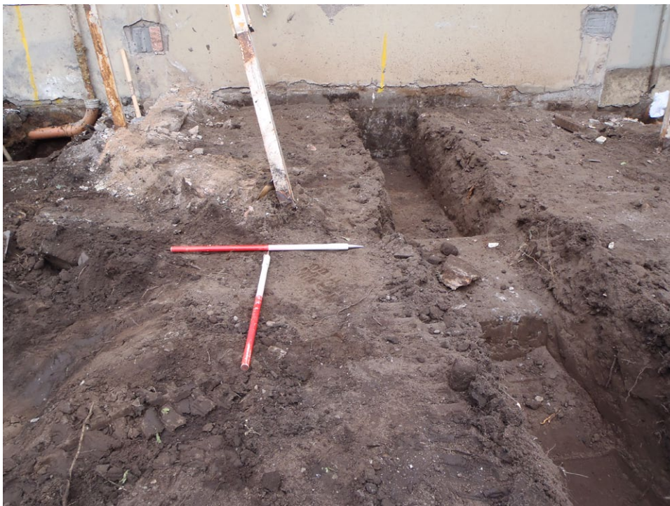
Fig. 5 - Remains of modern conservatory foundations on northern side of trenches adjoining existing house
