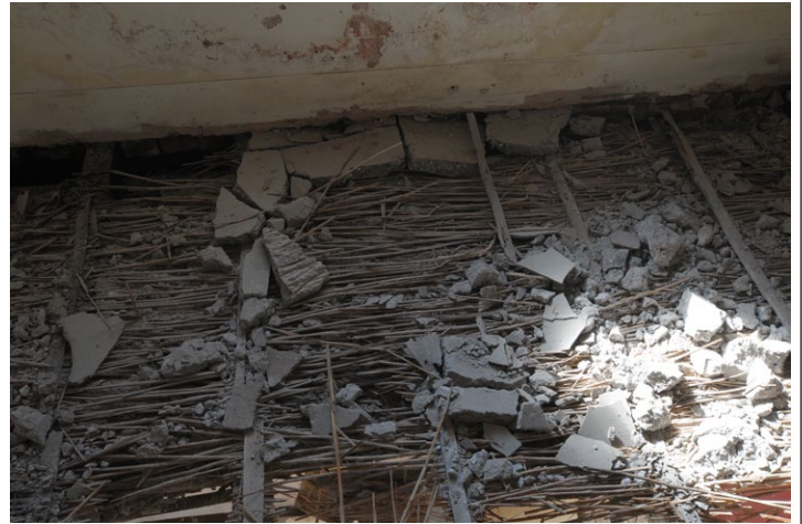
Fig. 26 - Close up of reed and concrete floor, west room, 1st floor, Unit 1, looking south
