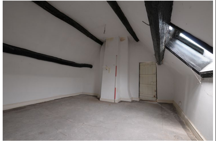
Fig. 32 - Shot showing fireplace in east room, 2nd floor (attic), Unit 1, looking north-east
