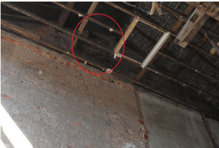
Fig. 33 - Blocked window at east end of Unit 1 attic, shot taken from Unit 2, view north-west
