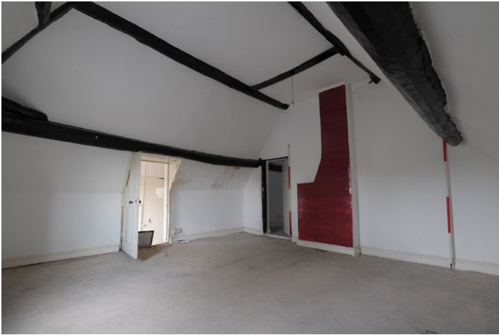
Fig. 31 - Shot showing fireplace in west room, 2nd floor (attic), Unit 1, looking north-east
