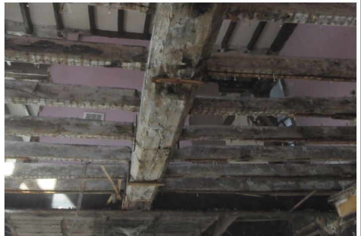
Fig. 16 - Shot of original beam in ceiling, ground floor (east side) Unit 1, looking west
