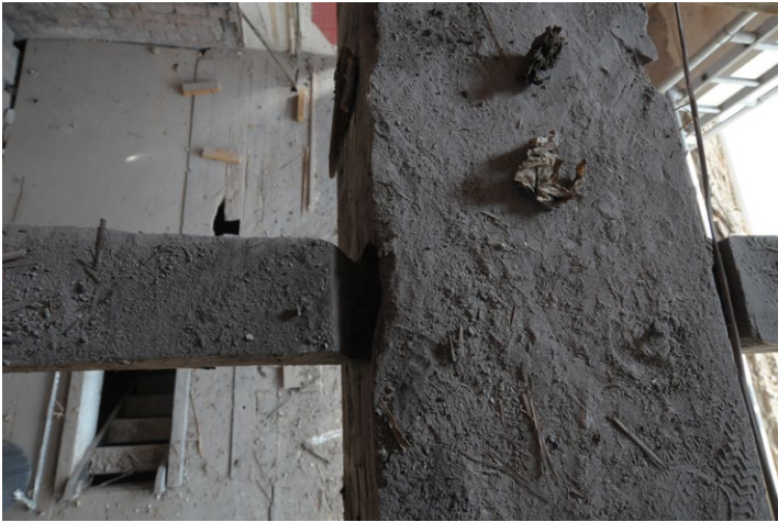
Fig. 25 - Close-up of slot in beam for joist and newspaper inserted into remaining void, east room, 1st floor, Unit 1, looking east
