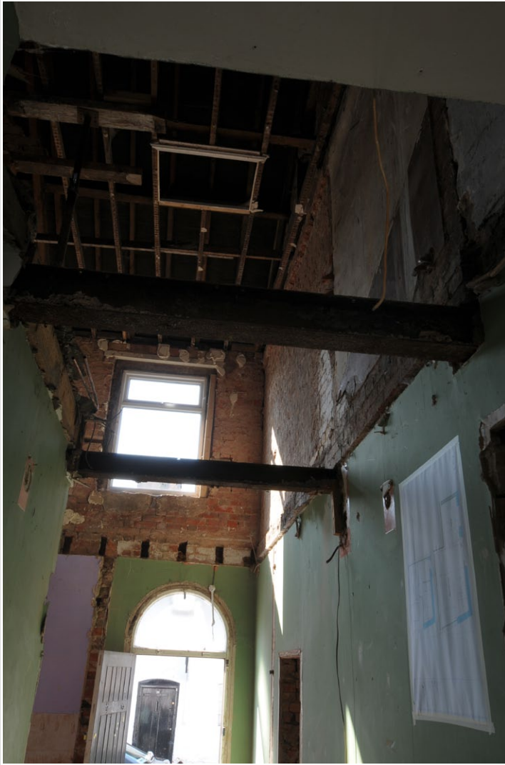
Fig. 37 - Internal view of lower floor of Unit 2 after ceiling removed, looking South
