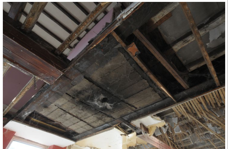
Fig. 18 - Photo of concrete and steel beams holding up chimney above ground floor, Unit 1
