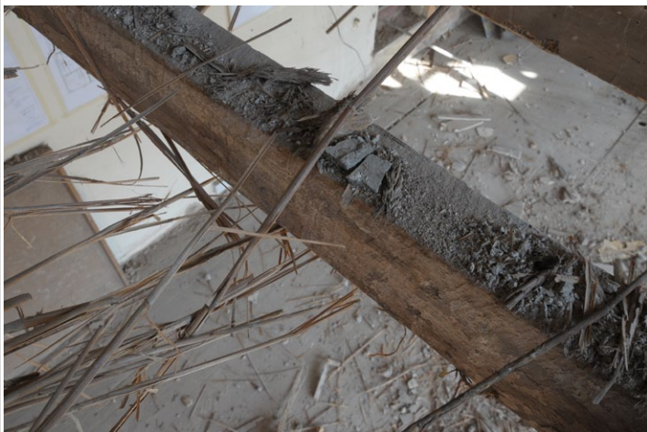
Fig. 23 - Shot of pit sawn floor joist, west room, 1st floor, Unit 1, looking north-east
