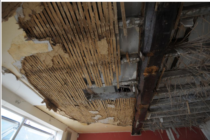
Fig. 17 - Shot of original beam in ceiling, ground floor (west side) Unit 1, looking west
