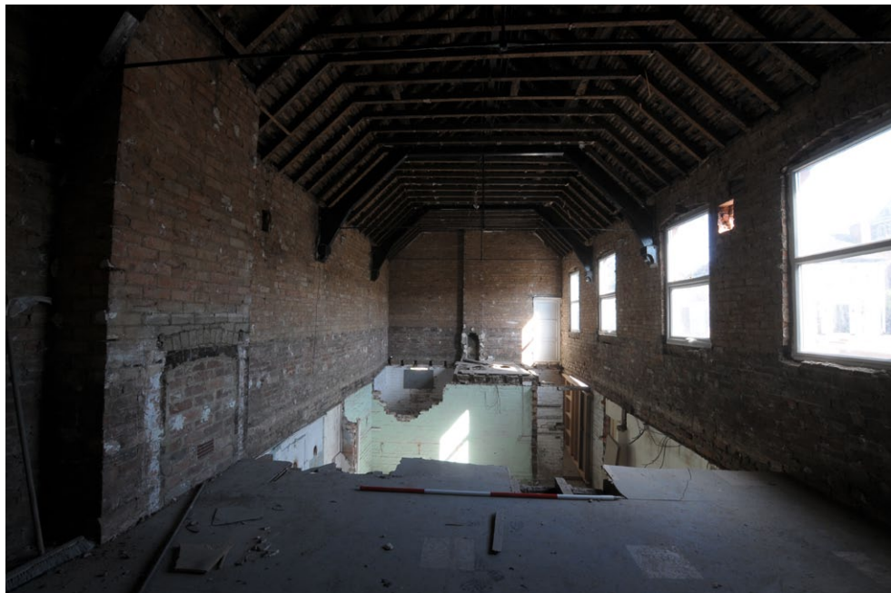
Fig. 45 - Internal view of upper floor of Unit 4 after floor partially removed, looking north
