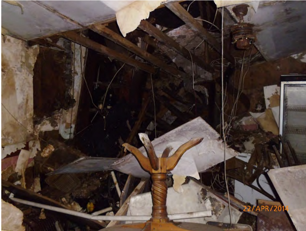
Plate 11: Interior condition of No.13 Dalry Rd (taken by client)
