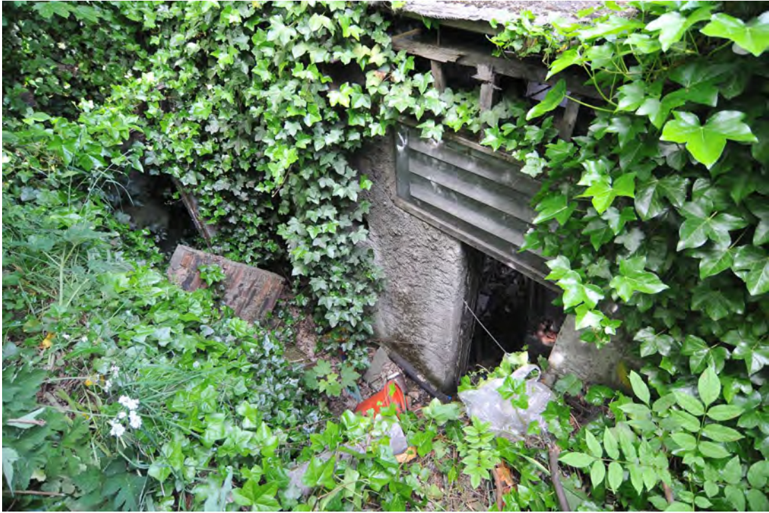
Plate 7: View of back yard and overgrown steps
