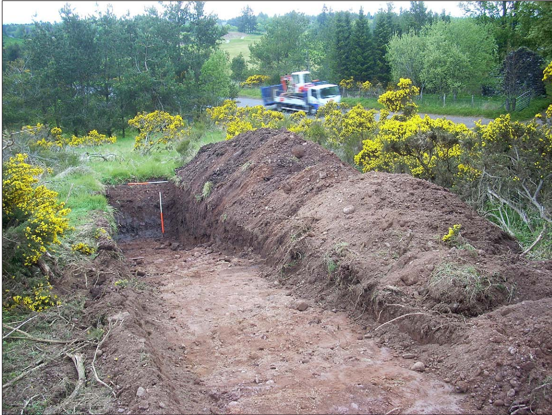
Fig. 12 - Trench 20. Break of slope at the northern end where the natural subsoil has been truncated by the cutting for the underpass
