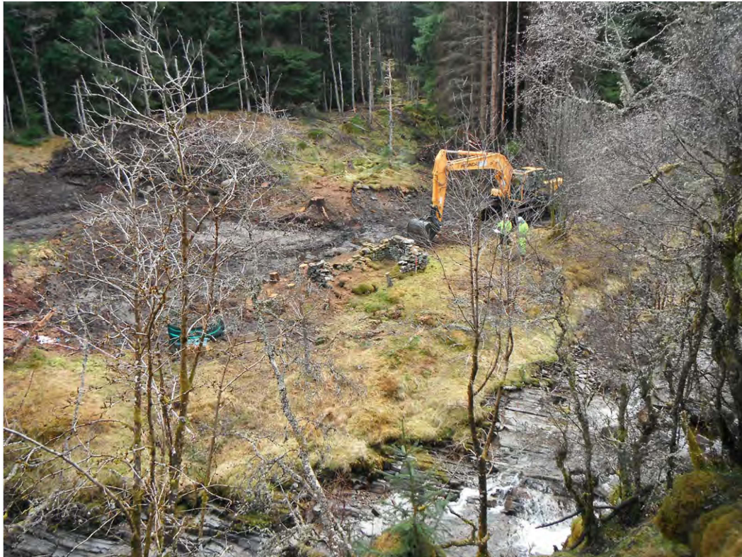
Fig. 5 General view of the Intake 1 area from the west post-felling. Sites 4a and 4b are just to the left of the digger
