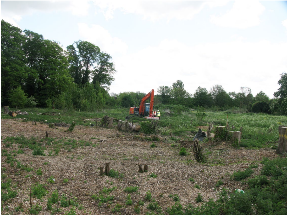
Fig. 4 - General shot of the site from the north-west showing cut down trees.
