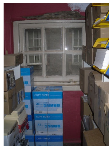
View of crumbling plasterwork around window.
