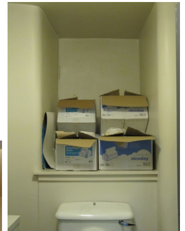
Deep recess behind toilet facility
