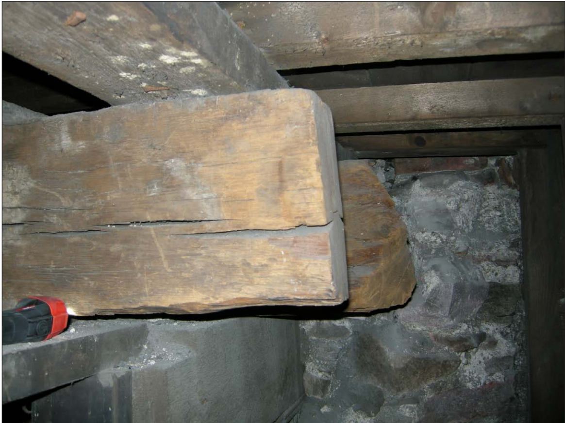
Plate 9 - North Block, north side, one of three re-used oak beams carrying the timbers for the flat roof
