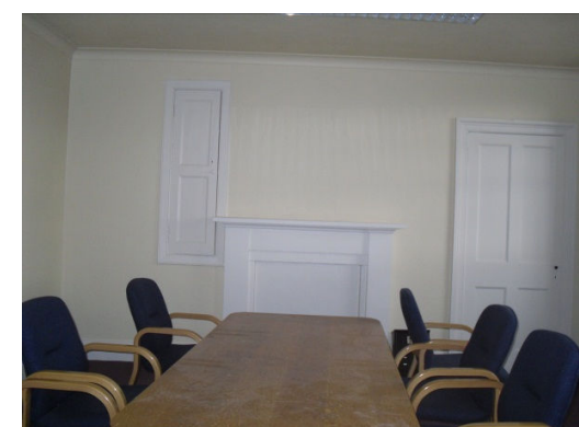
View of S.11 facing east wall, with high cupboard door on left, blocked fireplace in centre and press on right.
