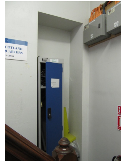
Recess in wall, was former door giving access to this part of the building.
