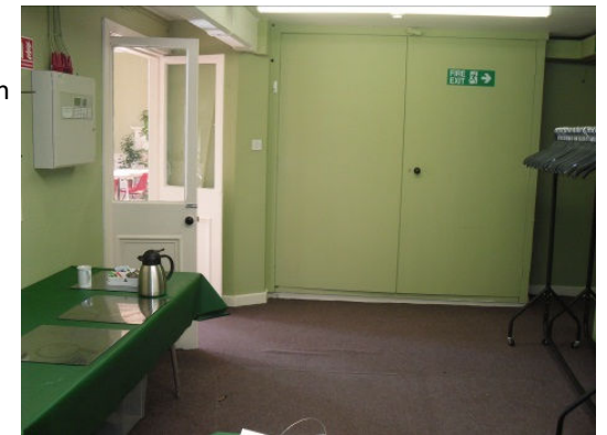
View of G.07 facing west , with distribution boards in cupboard ahead.
