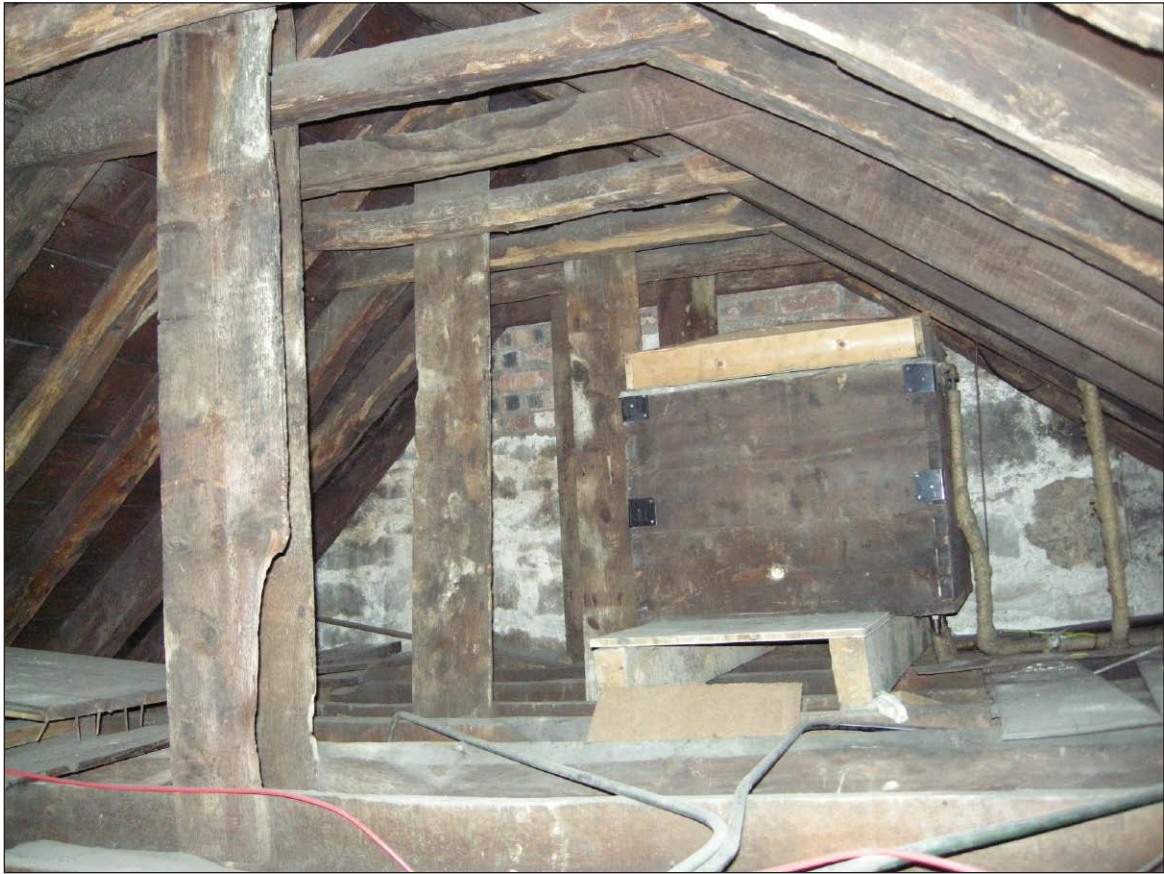
Plate 1 - South Block, general view of the A-frame roof trusses at the west end
