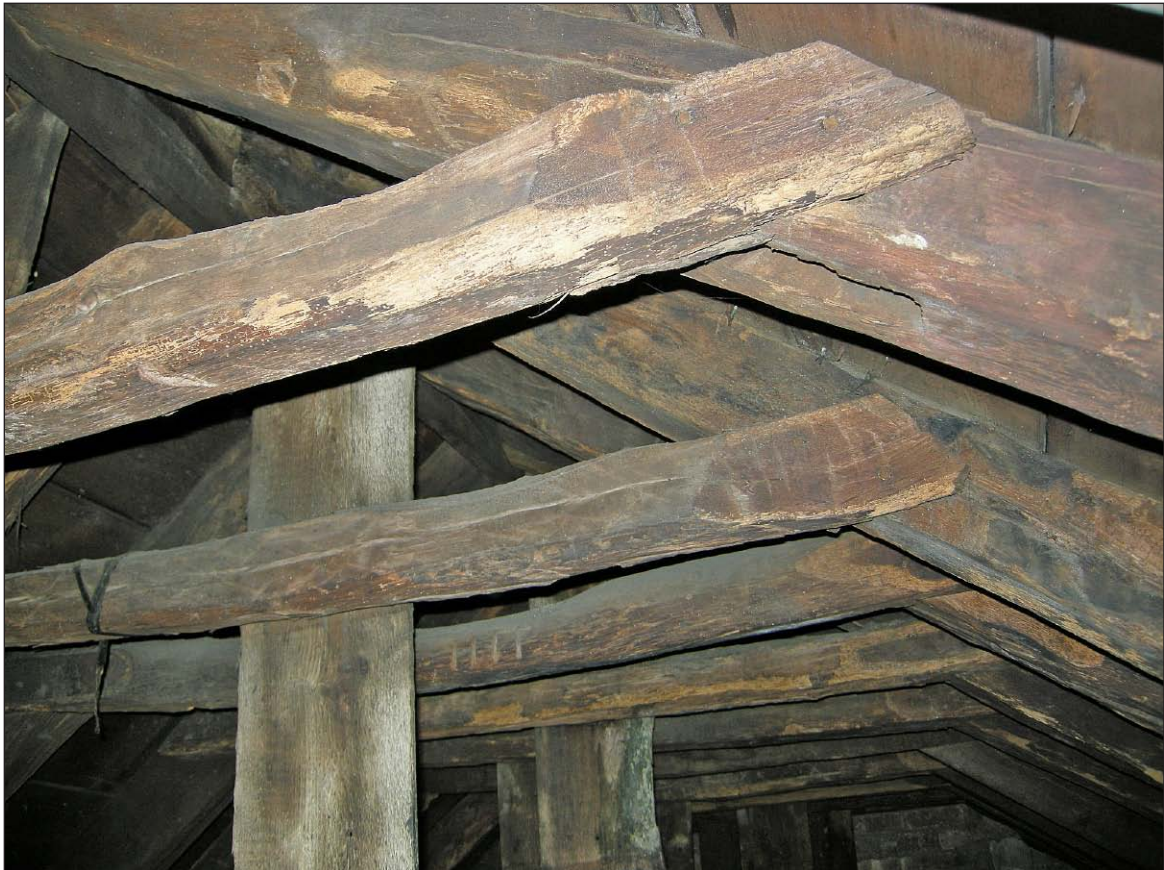
Plate 2 - South Block, close up of the rafter collars showing lap jointing onto the principal rafters
