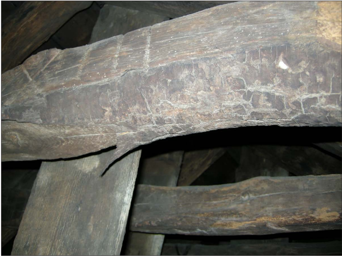
Plate 3 - South Block, close up of a numbered pine collar with bark in situ
