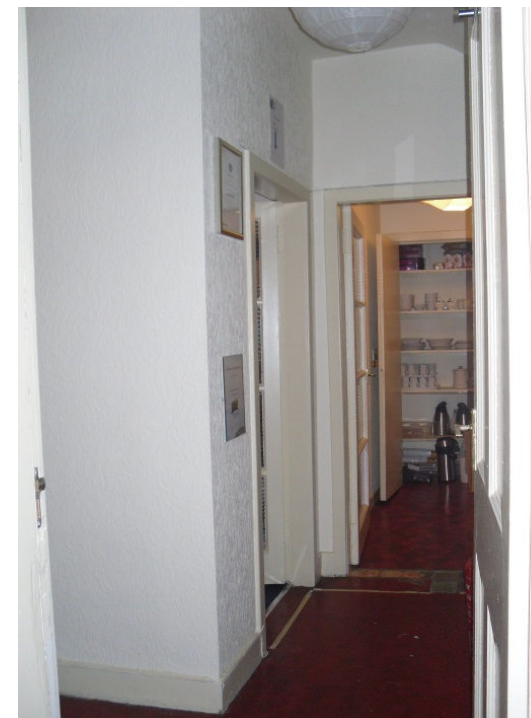
View of S.16, with first left leading to S.20 and kitchen straight ahead. Evidence of worn laminate floor in front of kitchen entrance.
