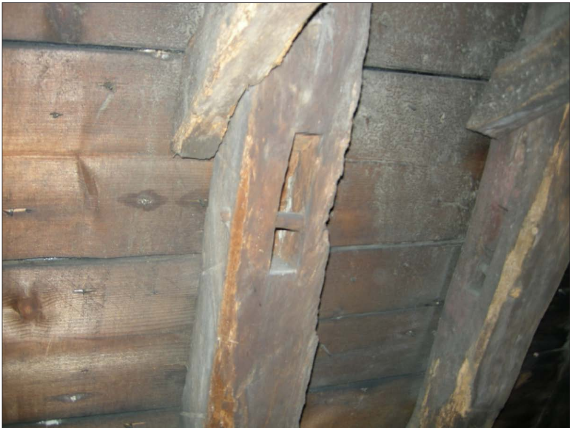
Plate 4 - South Block, detailed shot of a mortise joint with a peg still in situ, note the neighboring rafter with a mortise joint at the wrong angle
