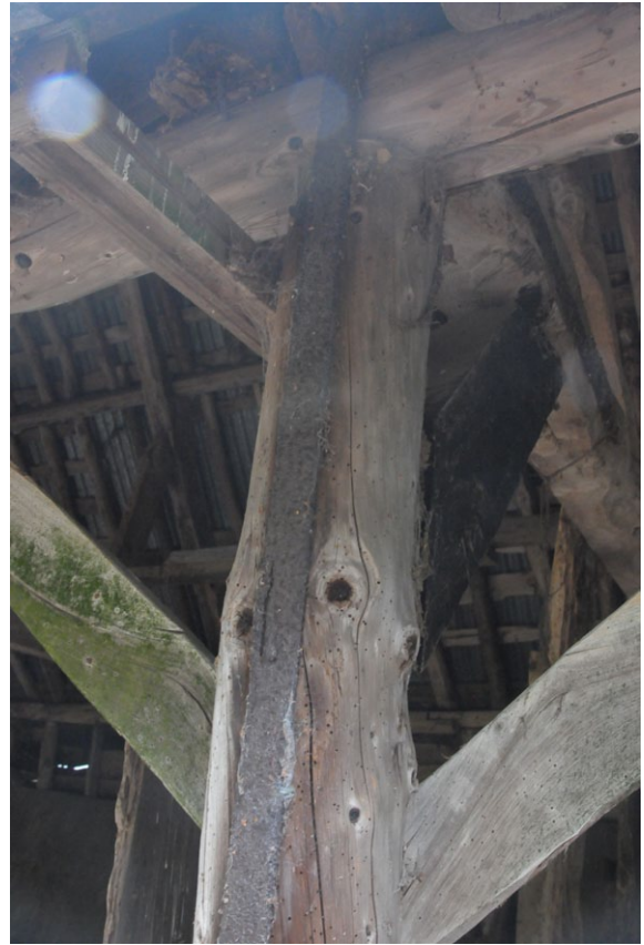
Fig. 32 - Iron strap joining the post, bressumer beam and tiebeam, east post, front elevation
