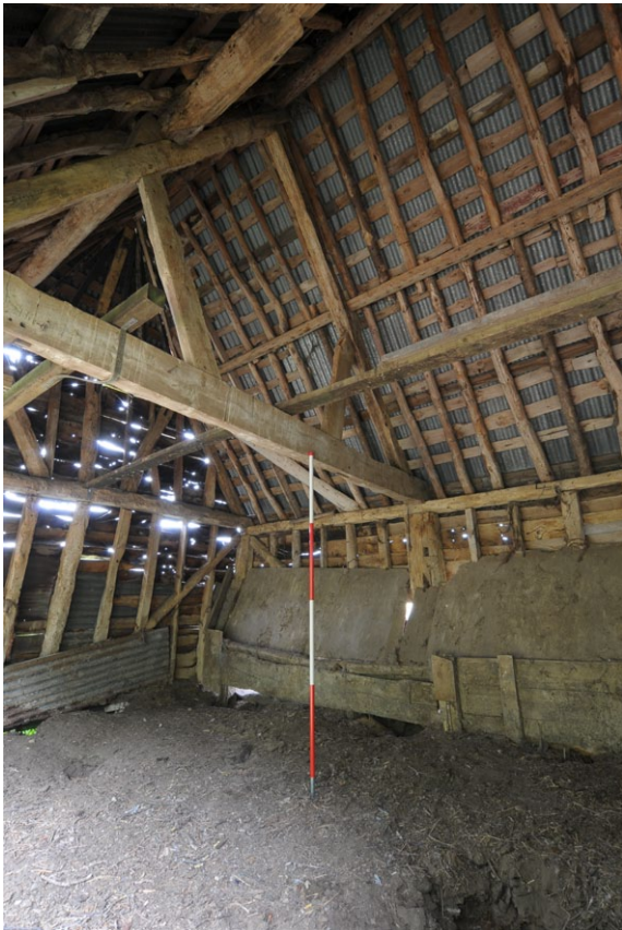
Fig. 12 - Shot of interior showing boarded up animal feeding trough
