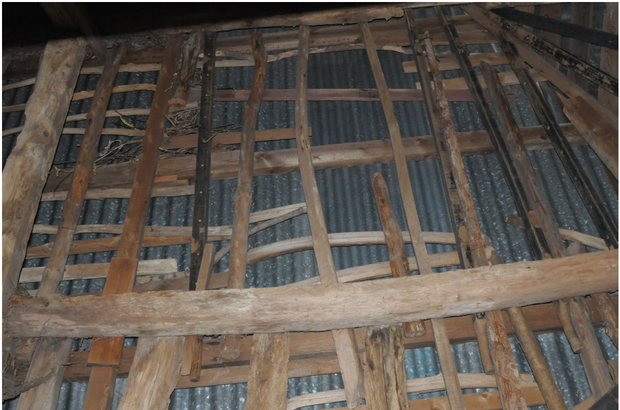
Fig. 30 - Split laths at west end of south pitch
