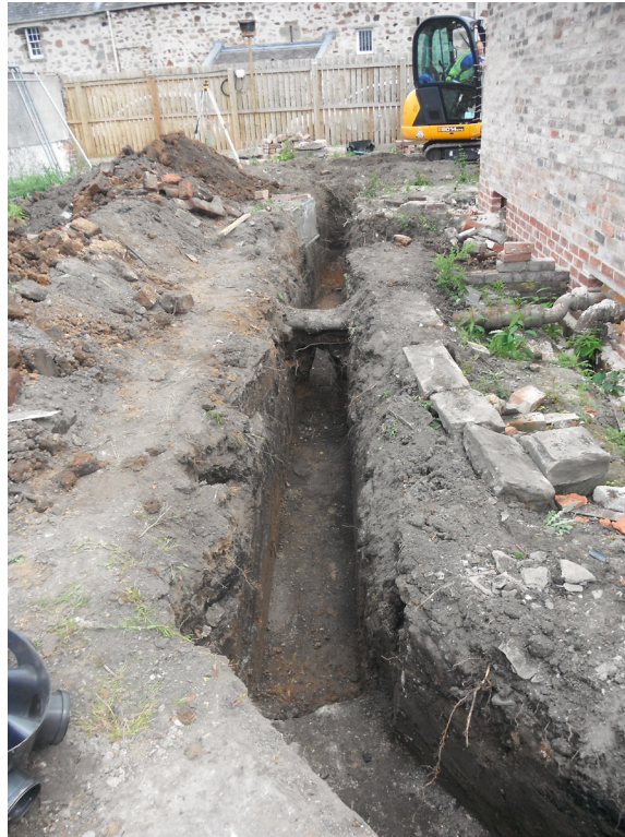
Fig. 3 Photograph of drainage trench on the northern side of greenhouse, from the west
