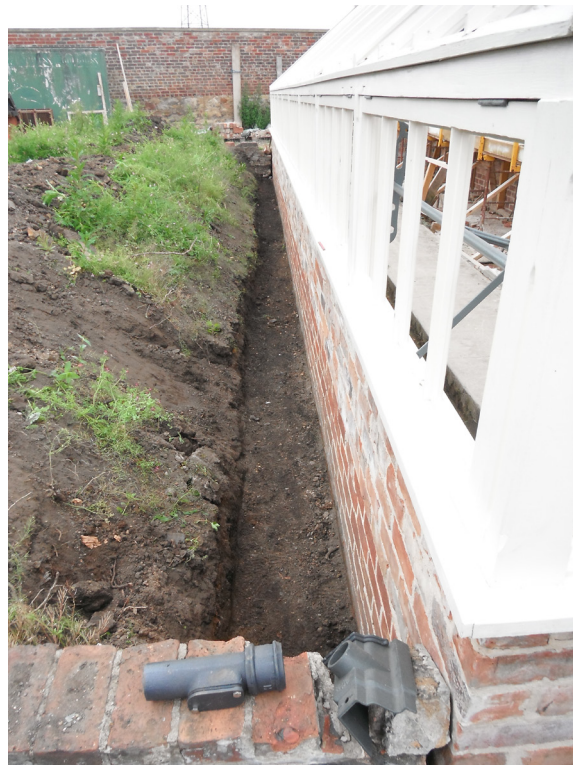
Fig. 4 Photograph of drainage trench on the southern side of greenhouse, from the east
