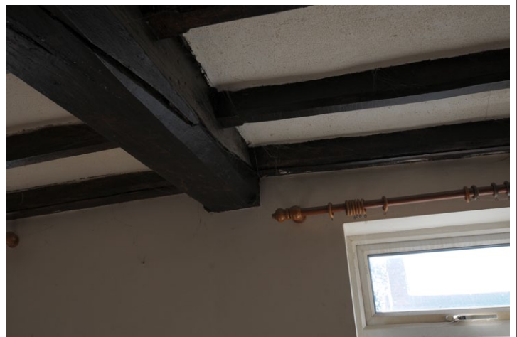
Fig. 30 - Shot of beam supporting attic floor, west room, 1st floor, Unit 1, looking south-east
