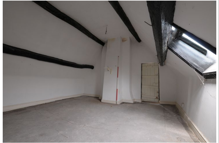
Fig. 32 - Shot showing fireplace in east room, 2nd floor (attic), Unit 1, looking north-east
