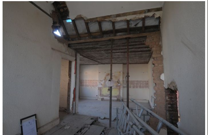
Fig. 41 - Internal view of upper floor of Unit 3 after stripping and wall demolition, looking east
