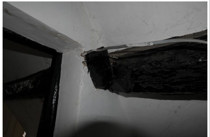
Fig. 34 - Splayed scarf joint for hewn purlins on north pitch of roof, 2nd floor (attic), Unit 1, looking north-west
