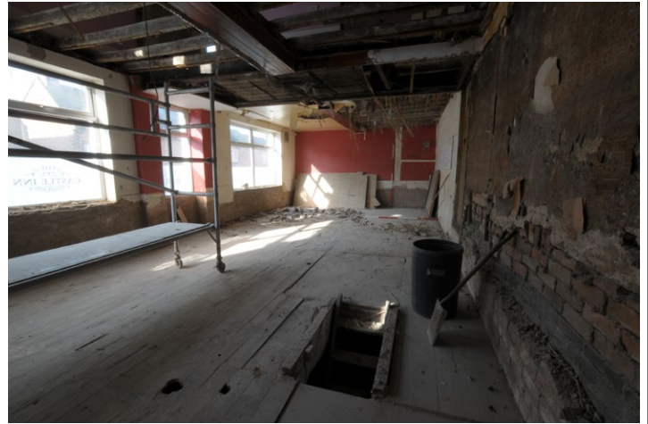
Fig. 14 - General shot of ground floor after walls and ceiling stripped, Unit 1, looking west
