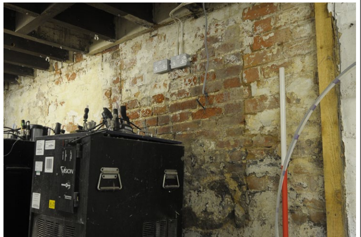
Fig. 49 - Original bricks above stone foundations, Cellar, Unit 1, looking north-west. Patching of walls in later brick can be seen on either side
