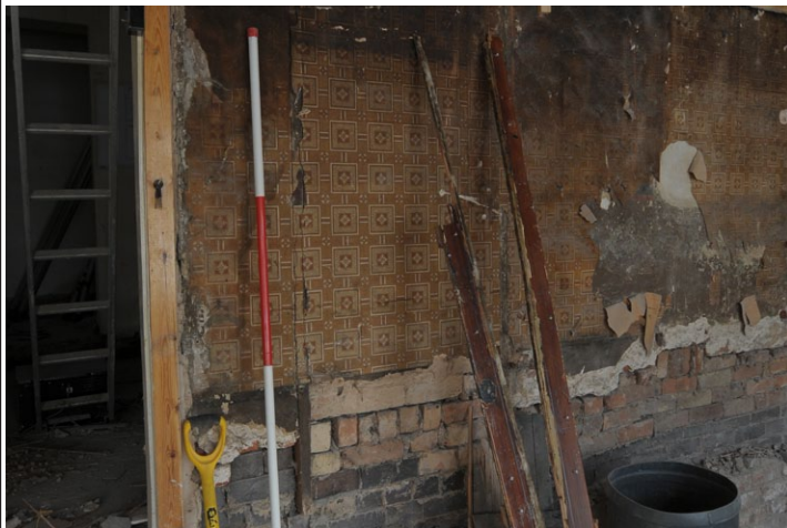
Fig. 15 - Shot of blocked doorway in north wall, ground floor, Unit 1, looking north
