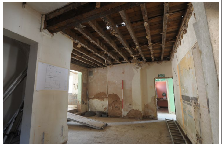
Fig. 39 - Internal view of lower floor of Unit 3 after ceiling and walls stripped, looking east
