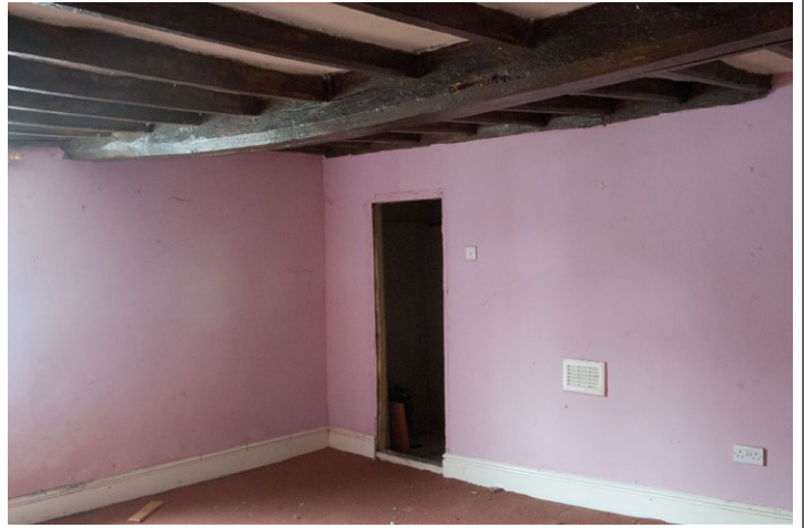
Fig. 20 - Shot of east room prior to floor being removed, 1st floor, Unit 1, looking south-west
