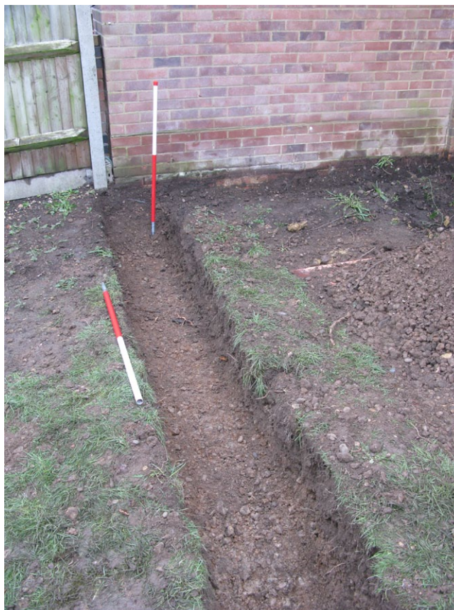
Fig. 3 - Northern end of western foundation trench excavated to natural gravels, view looking NE
