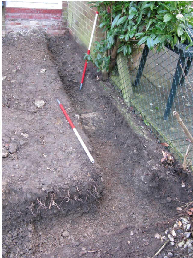
Fig. 4 - Southern foundation trench excavated to natural gravels showing waste water service, view looking SE
