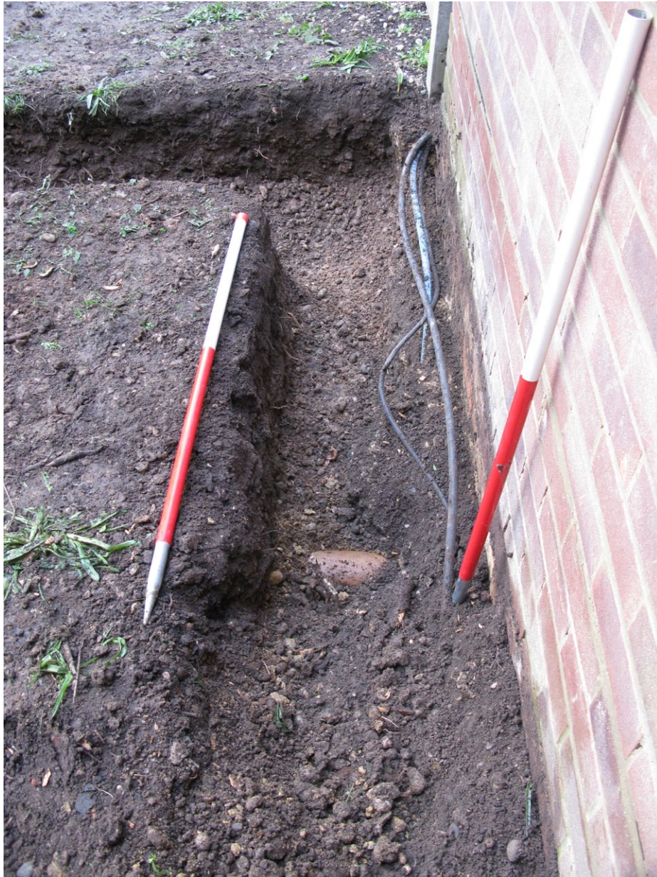
Fig. 6 - Northern foundation trench excavated to natural gravels showing waste water service, view looking W
