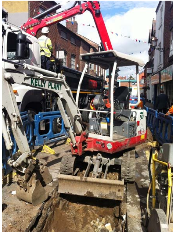
Plate 1: Working shot during the excavation of Pit 07, looking north along Princess Street
