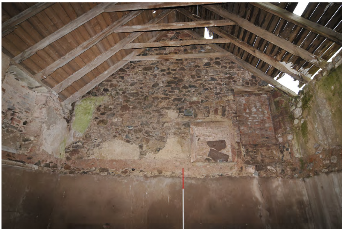
Fig. 23 Interior of the barn, Unit 23, with a blocked fireplace and window on the gable wall
