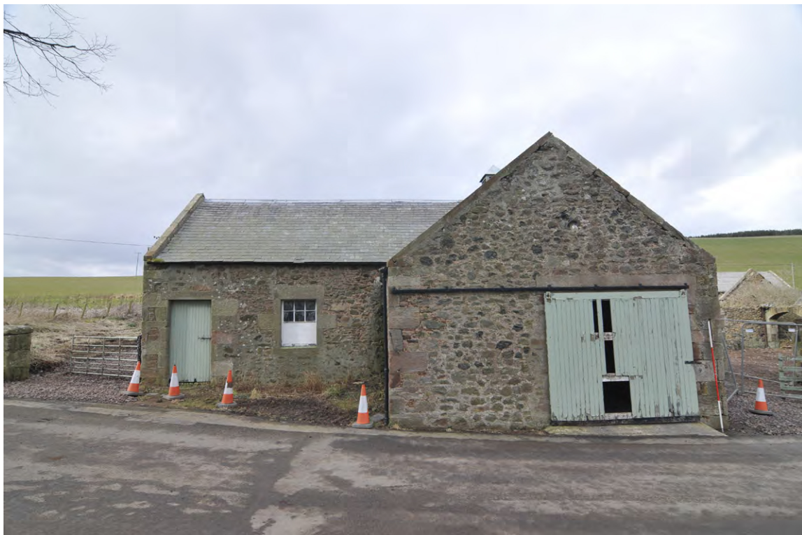
Fig. 11 South Range, west end, the gable of workshop/garage, Unit 31, and workshop, Unit 30
