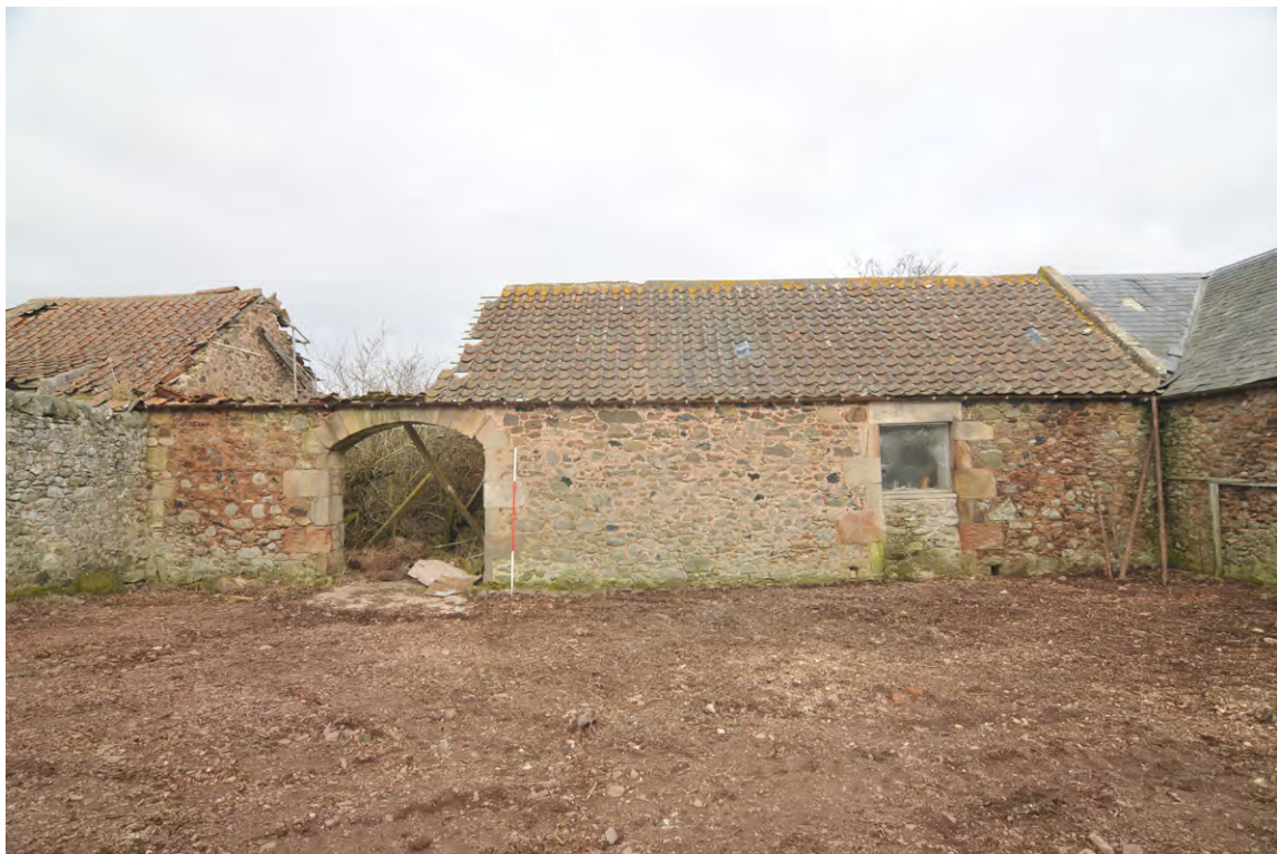
Fig. 9 East Range, west-facing elevation with collapsed byre roof in Unit 11
