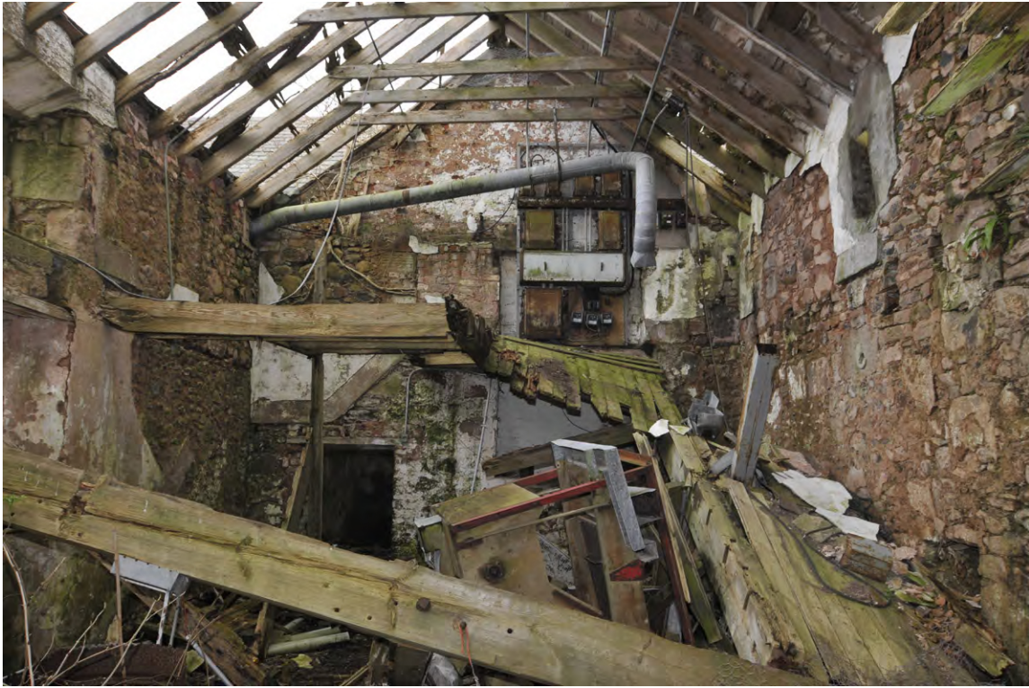
Fig. 20 Interior of the granary, Unit 20, with collapsed loft floor, a blocked fireplace can be seen to the left of the electrical switch gear
