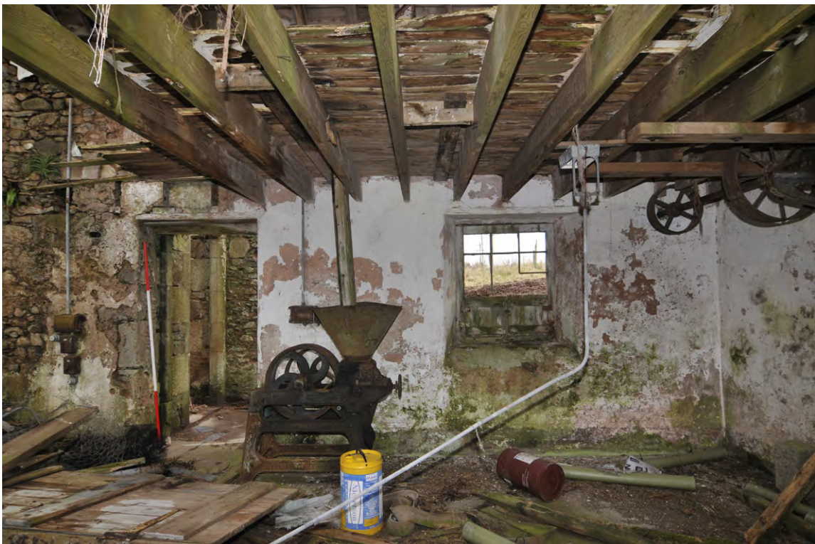
Fig. 21 Interior view of the granary with rear door and window. A belt driven oat crusher and belt drives can be seen
