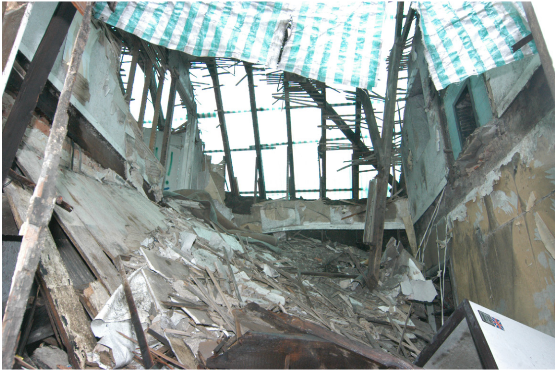
Fig. 10 Collapsed first floor and fireplace
