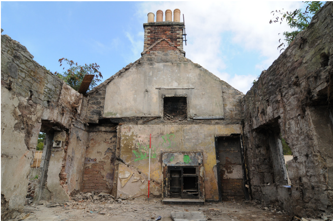
Fig. 23 Unit B, Southwest-facing elevation showing the partition wall with ground and first floor fireplaces
