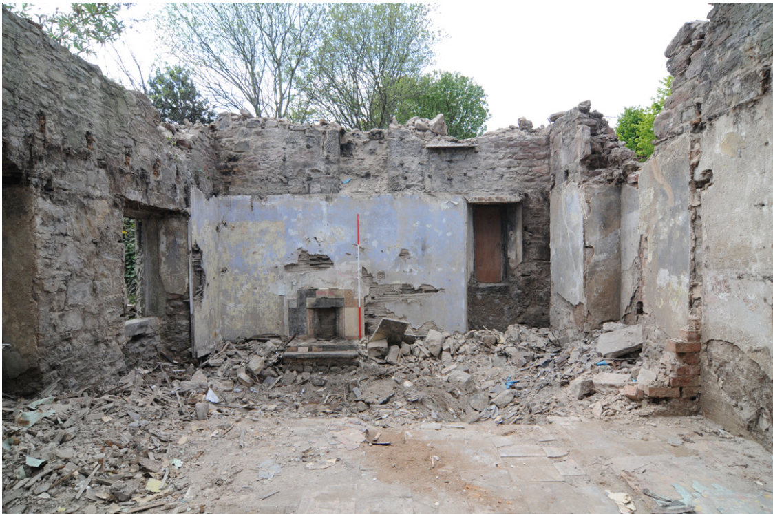
Fig. 21 Unit B, Northeast-facing elevation showing the reduced gable wall and fireplace
