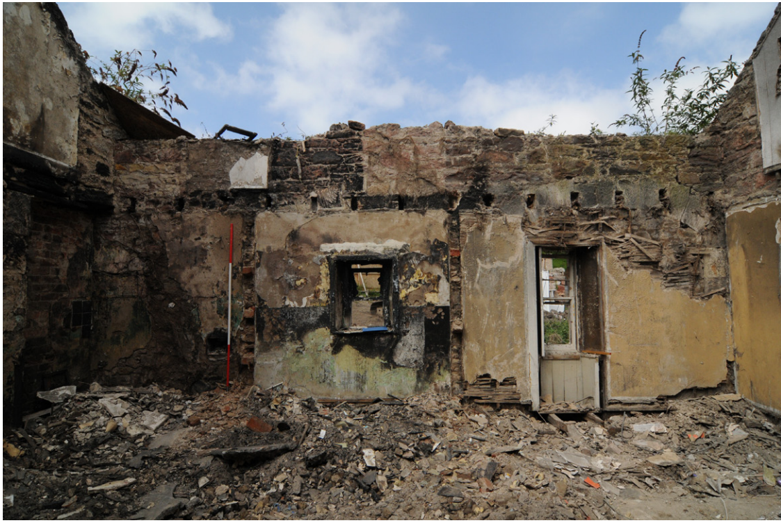
Fig. 18 Unit A, Southeast-facing elevation showing the interior of the blocked cart-shed openings
