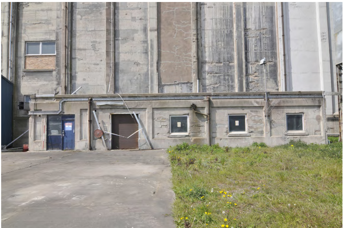
Fig. 13 Building D Grain Dryer Control Room
