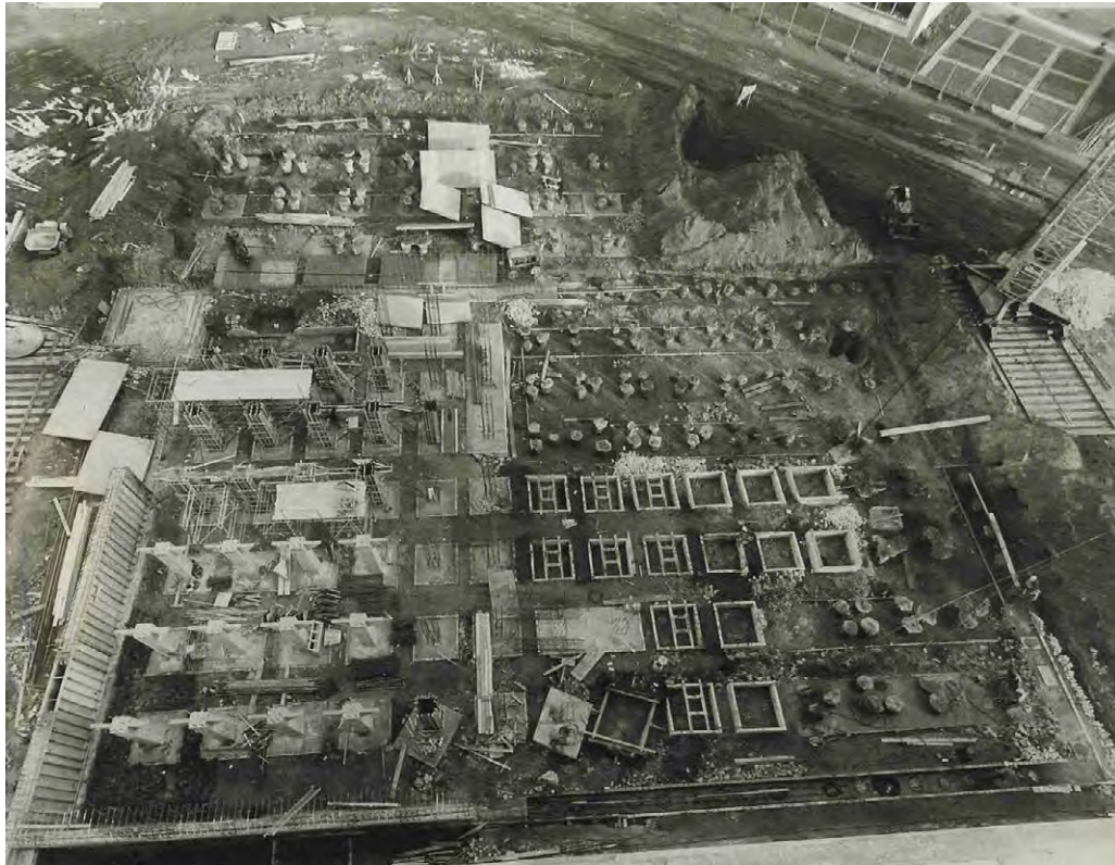
Fig. 20 Piling operations. Vertical view taken from the roof of the existing silos
