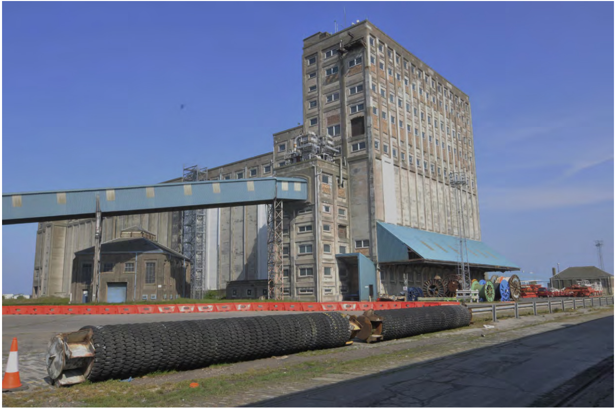
Fig. 6 Grain Conveyor incline to the weighing house on the west elevation
