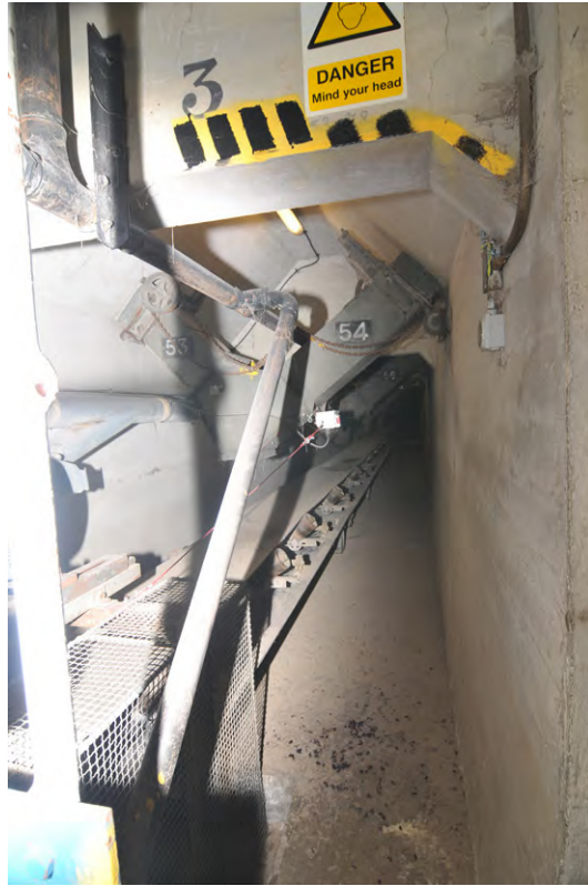
Fig. 30 Ground floor conveyor
