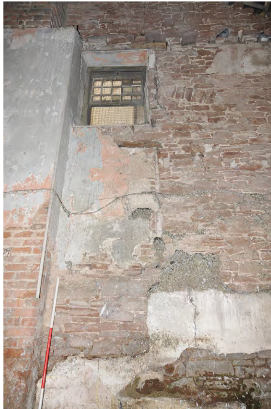
Fig. 9 Room 1, internal north-facing gable with small window and a blocked window below
