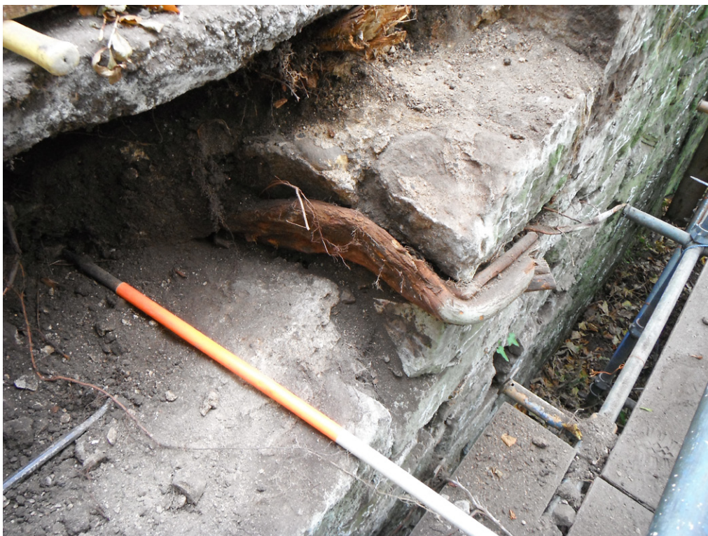
Fig. 5 - Tree roots (007) growing through the wall
