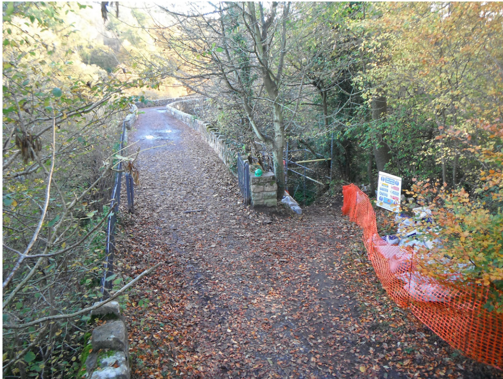
Fig. 2 - View from the north of the retaining wall location and the access over to the castle
