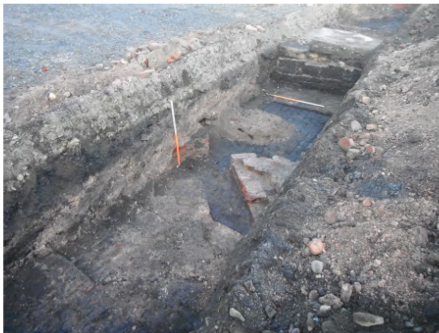
Fig. 46 - Mortar-bonded sandstone walls 906, 907, brick floor 910 and brick walls 908, 909 at the south-west end of the trench from the south-west
