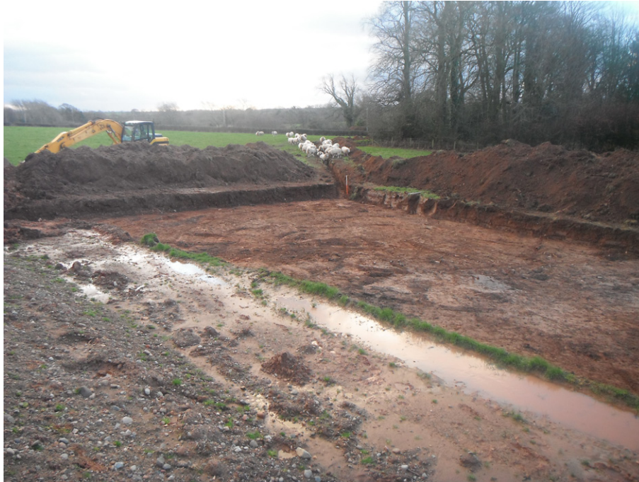
Fig. 20 - The northern portion of the electrical connection trench through the Scheduled Area from the north-west
