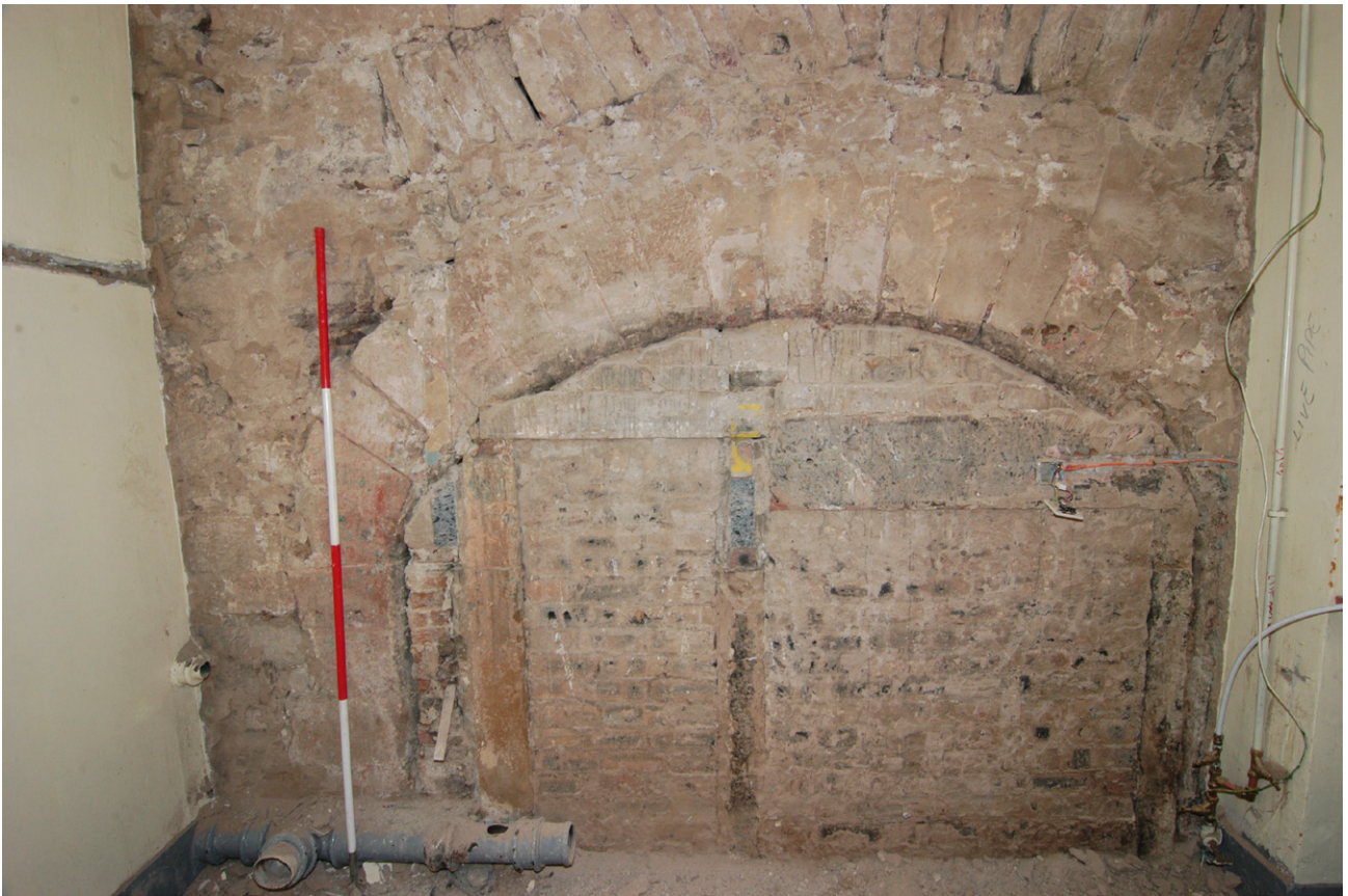
Fig. 13 - A large late 16th kitchen fireplace exposed following the removal of the wall plaster in Room G12, south-facing elevation
