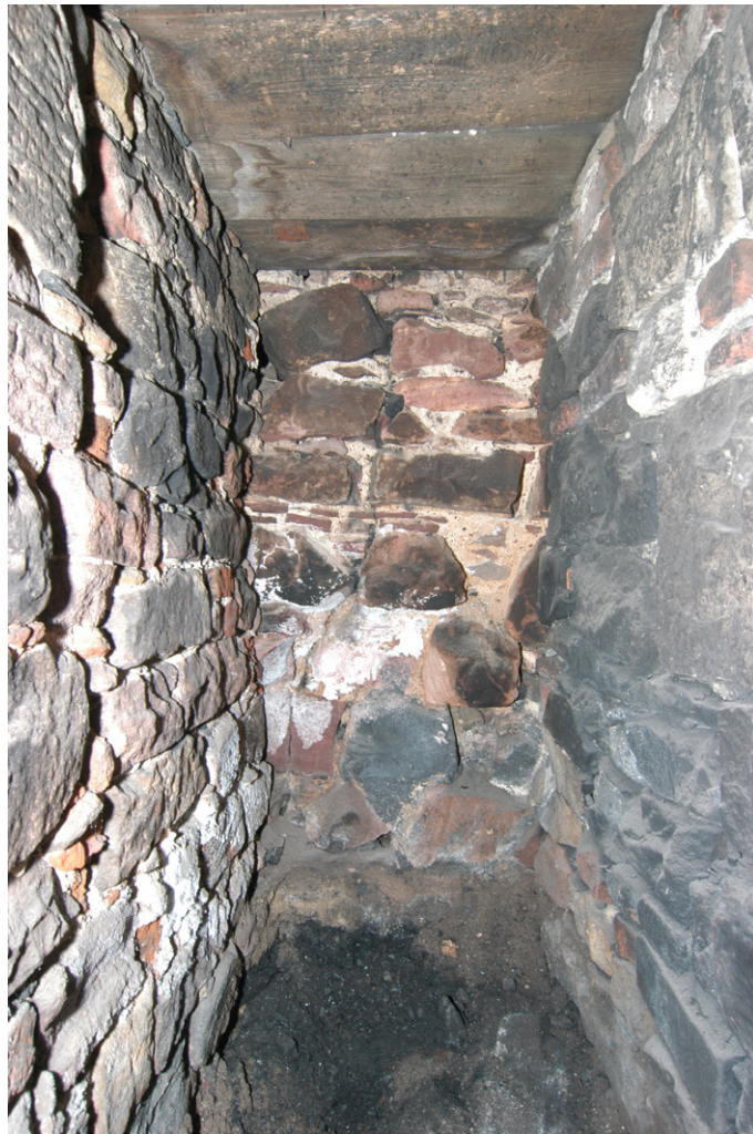
Fig. 14 - Interior of a 19th century coal cupboard in Room G12 after unblocking
