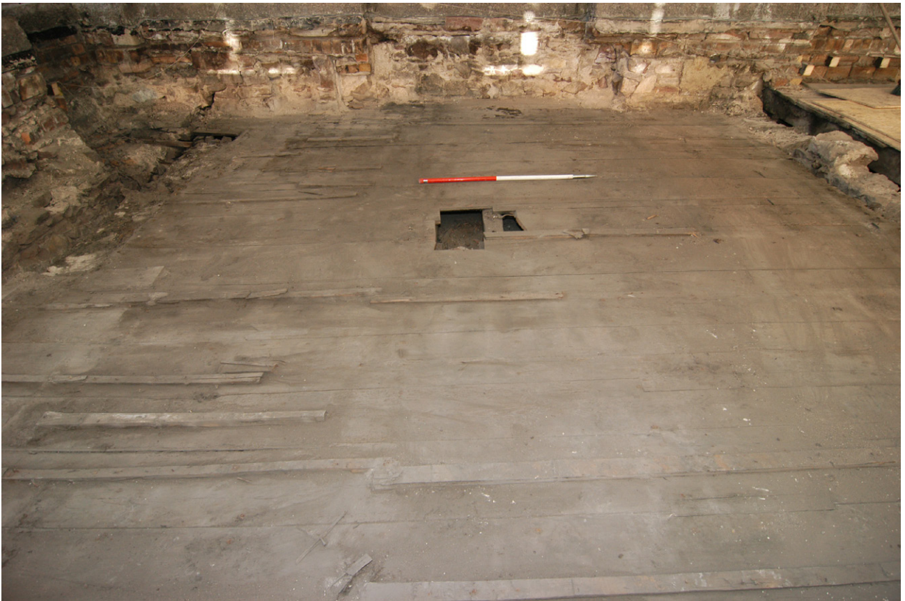
Fig. 34 - The floor boards in situ prior to uplifting on the North Block roof
