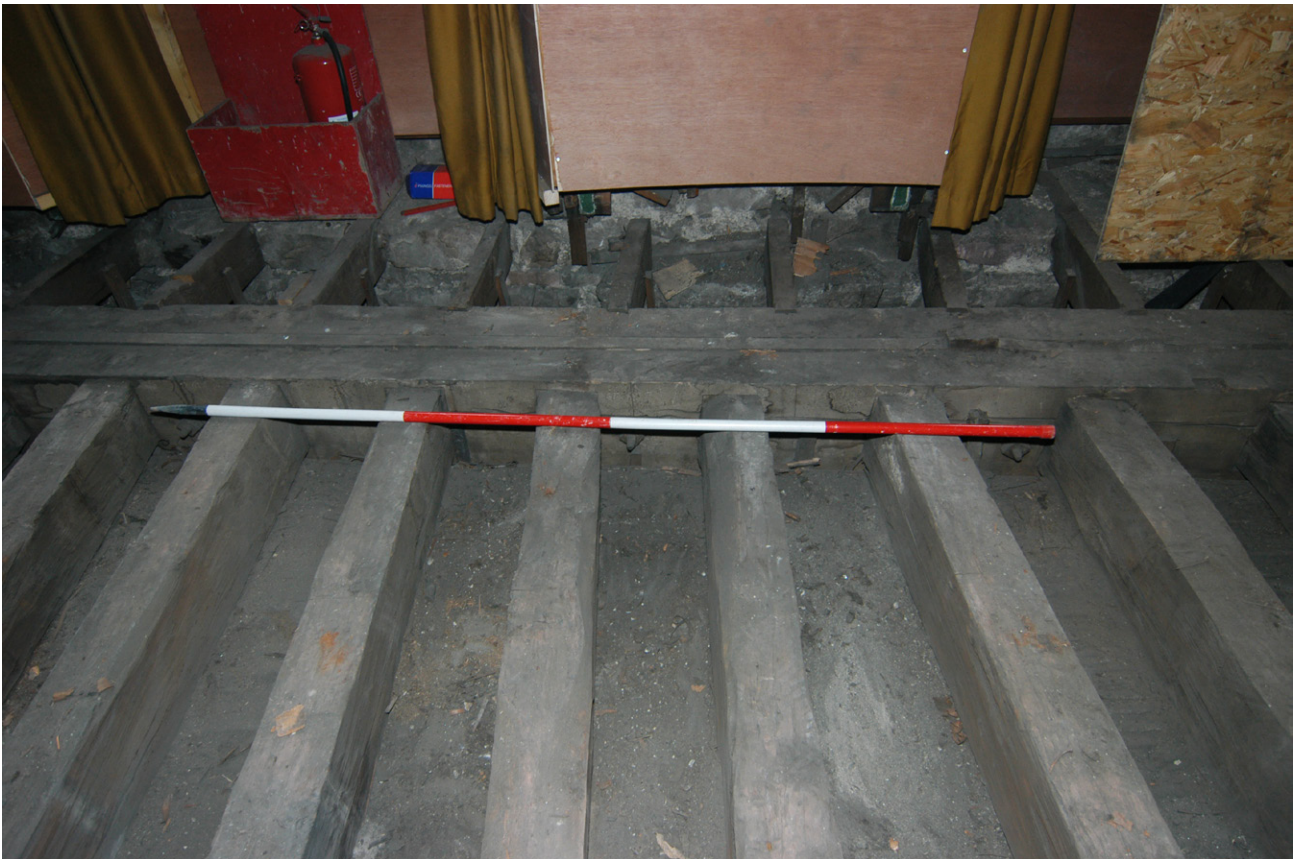
Fig. 25 - The oak floor joists and large flitch beam exposed in Room F09
