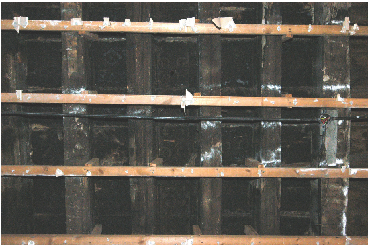
Fig. 29 - Exposed painted beams behind the battens of the modern ceiling in Room S02
