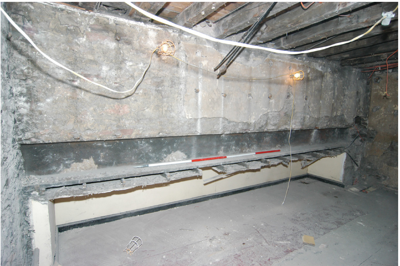
Fig. 28 - One of two 19th century Bressumer beams exposed within Room F12, north-facing elevation
