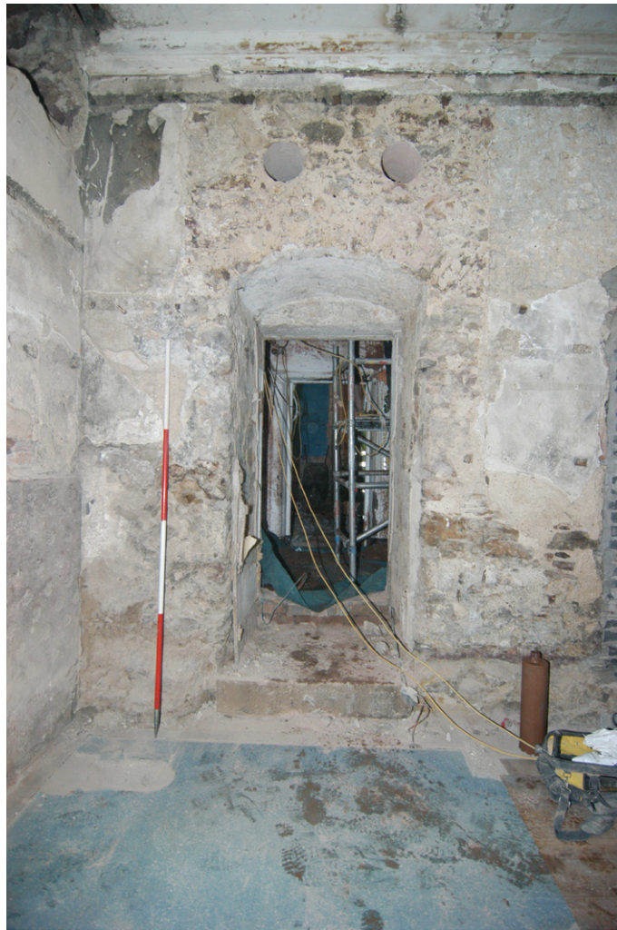
Fig. 5 - An early 16th century arched doorway in Basement Room B02 leading into a former vaulted cellar
