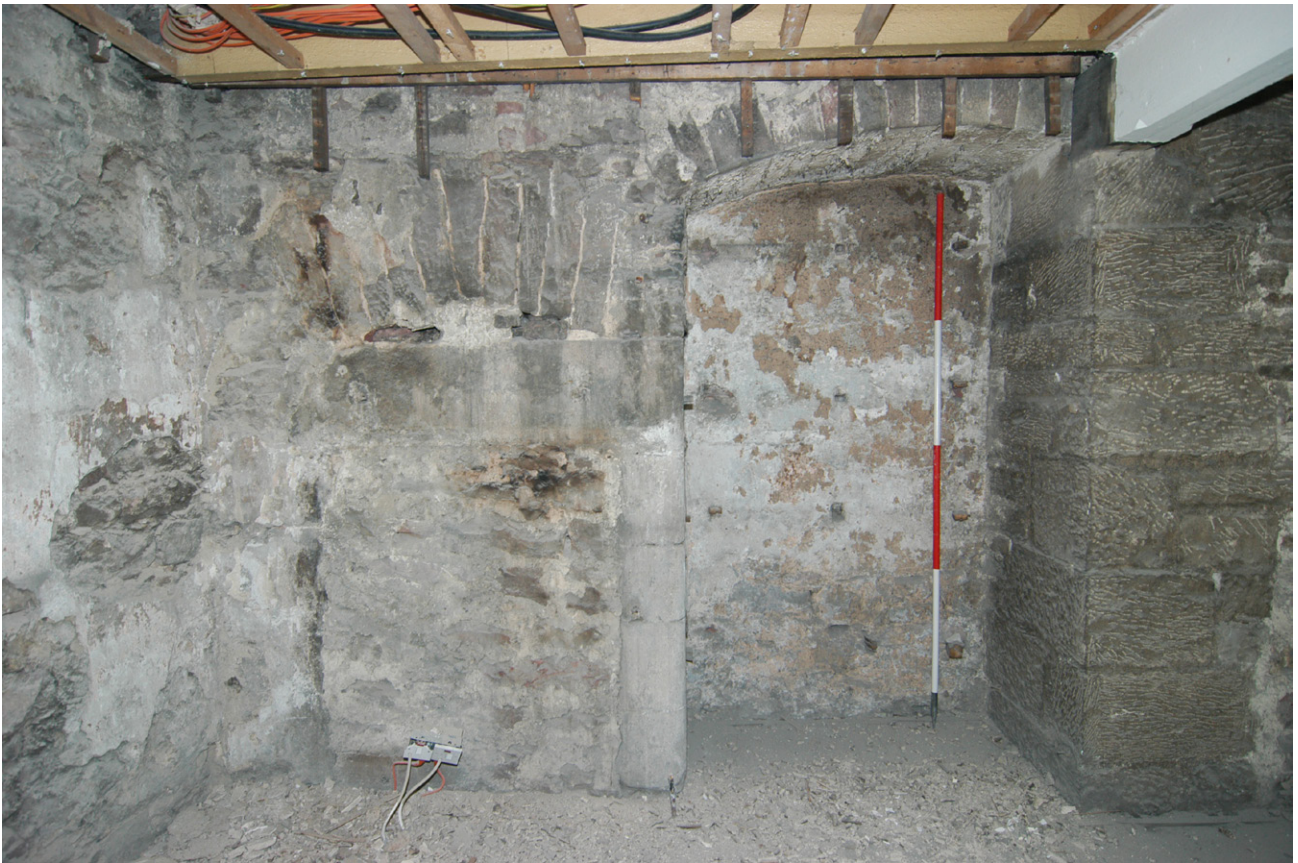
Fig. 12a - A blocked fireplace and press recorded in Room G07 west-facing elevation
