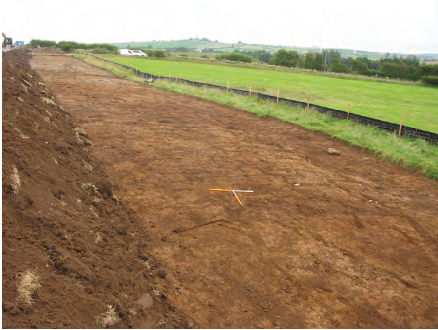
Fig. 11 - WA132, looking from the west along the stripped area for the wayleave
