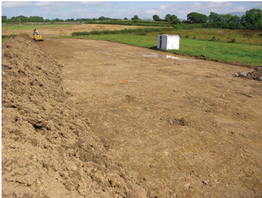
Fig. 12 - WA187, looking from the north-west along the stripped area for the wayleave
