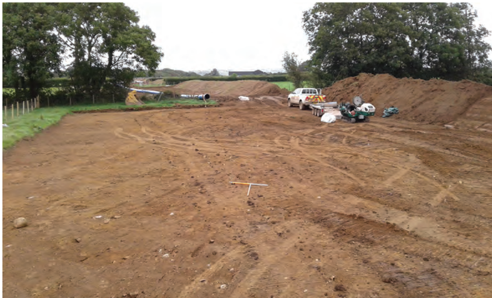
Fig. 10 - WA30, looking from the north-east along the stripped area for the wayleave
