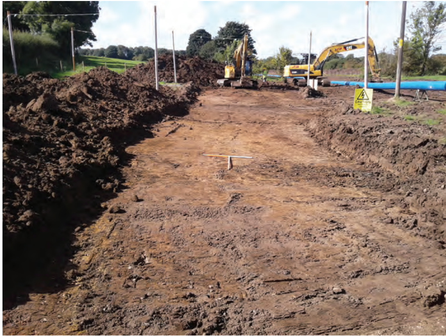
Fig. 13 - WA508, looking from the east-north-east along the stripped area for the wayleave
