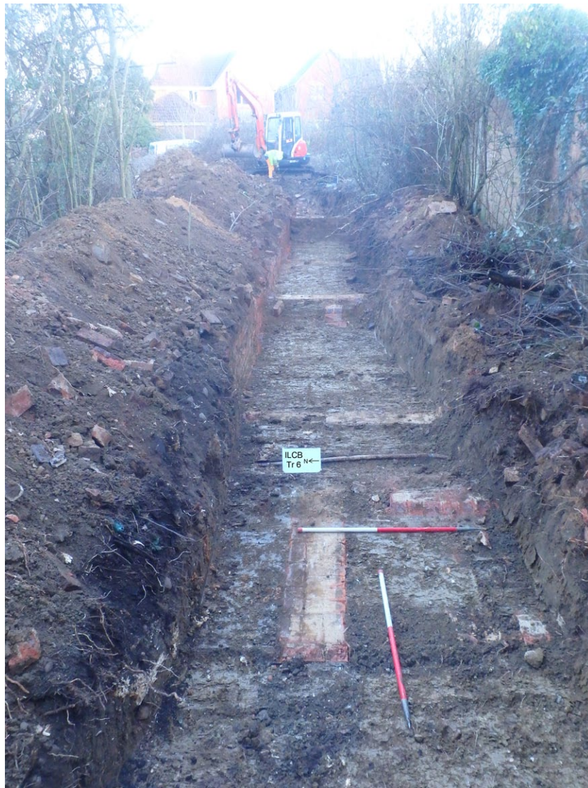
Fig. 14 - General view of Trench 6 showing building foundations north of upstanding wall, facing E
