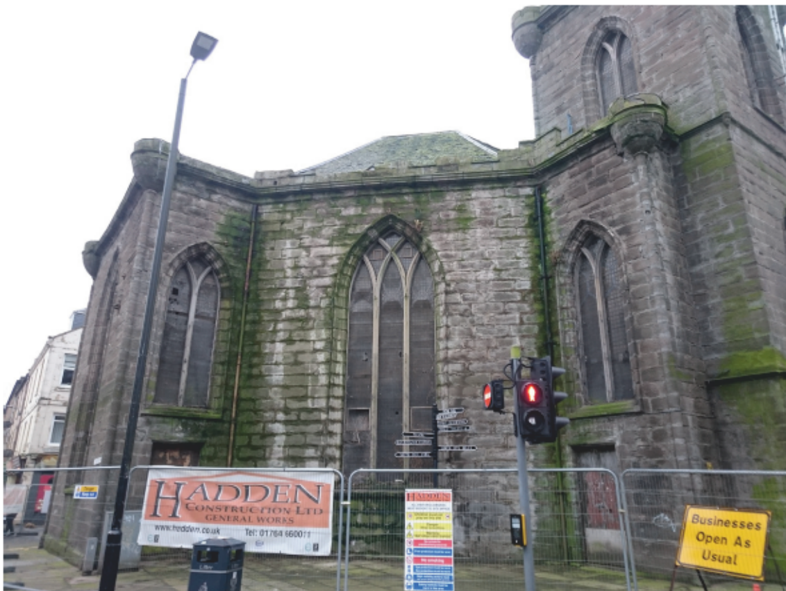
Fig. 6 - General view of the east-facing elevation and doorways before the scaffold was erected
