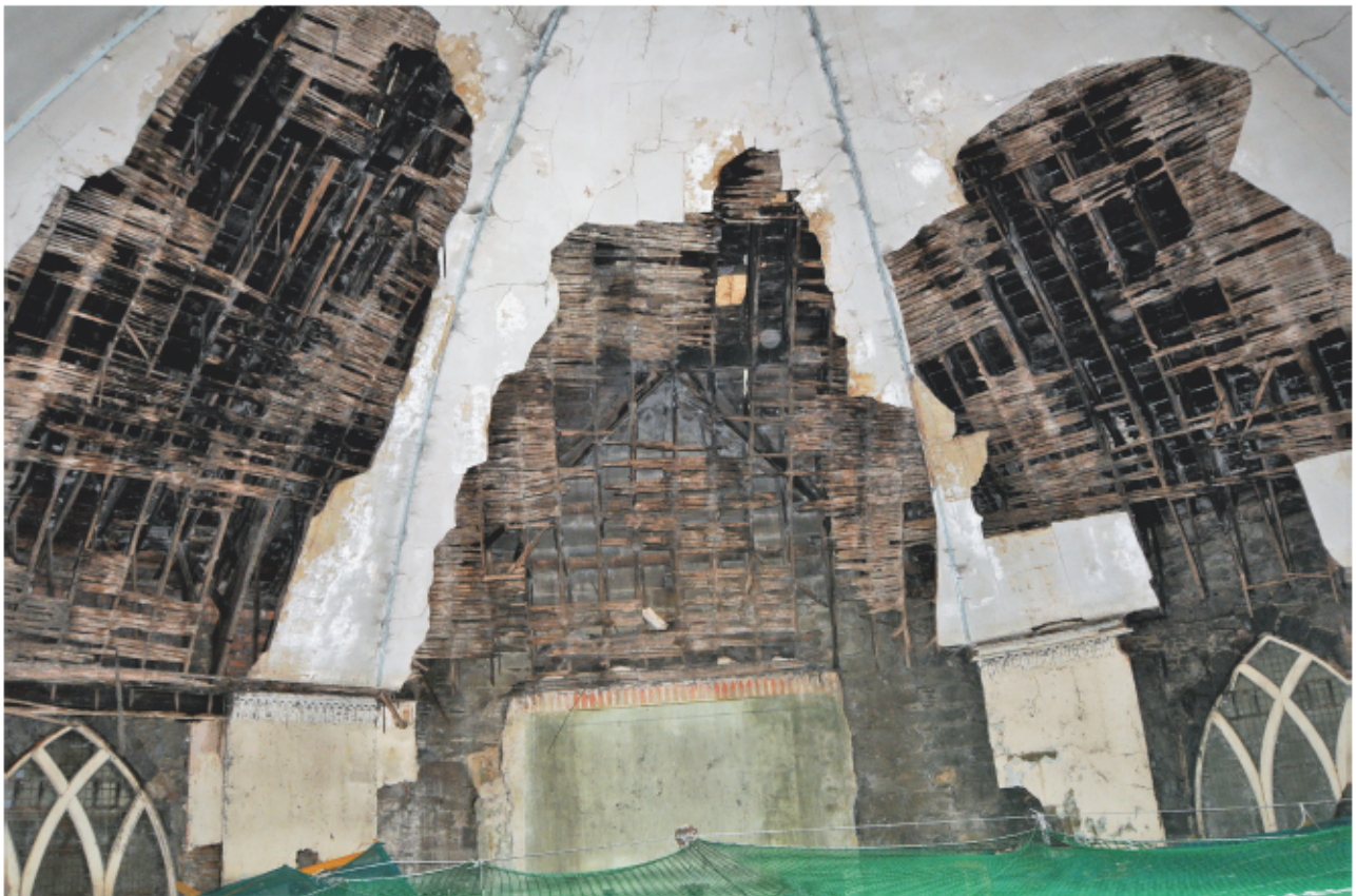
Fig. 28 - Part of the collapsed ceiling with exposed lath and plaster
