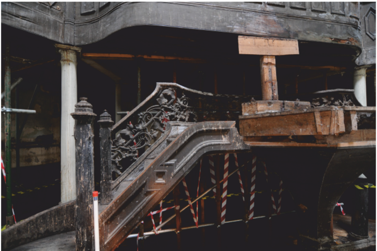
Fig. 15 - The remains of the pulpit with its missing ornate hand rail and strings (west side)
