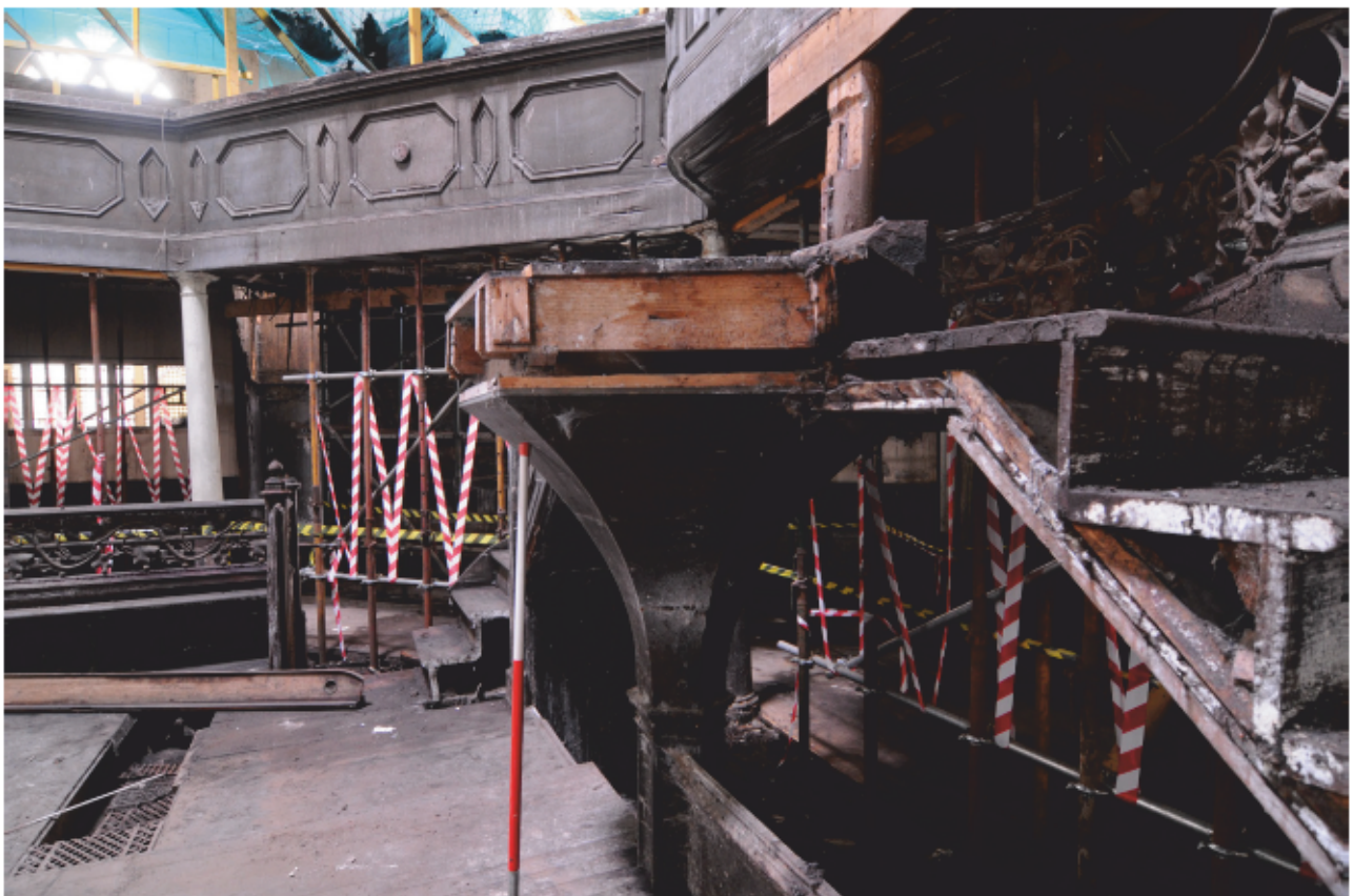
Fig. 14 - The remains of the pulpit with its missing ornate hand rail and frontage (east side)
