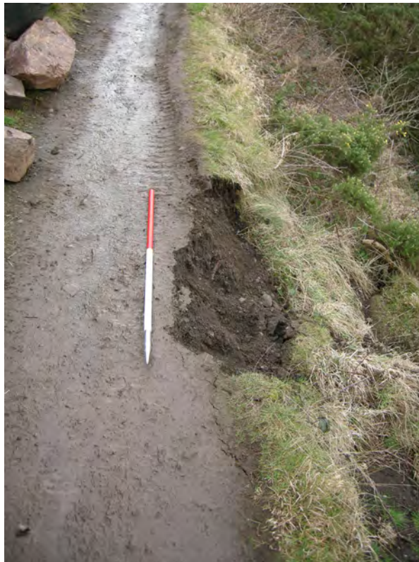
Fig. 13 - Path collapse due to snowmelt Area 3
