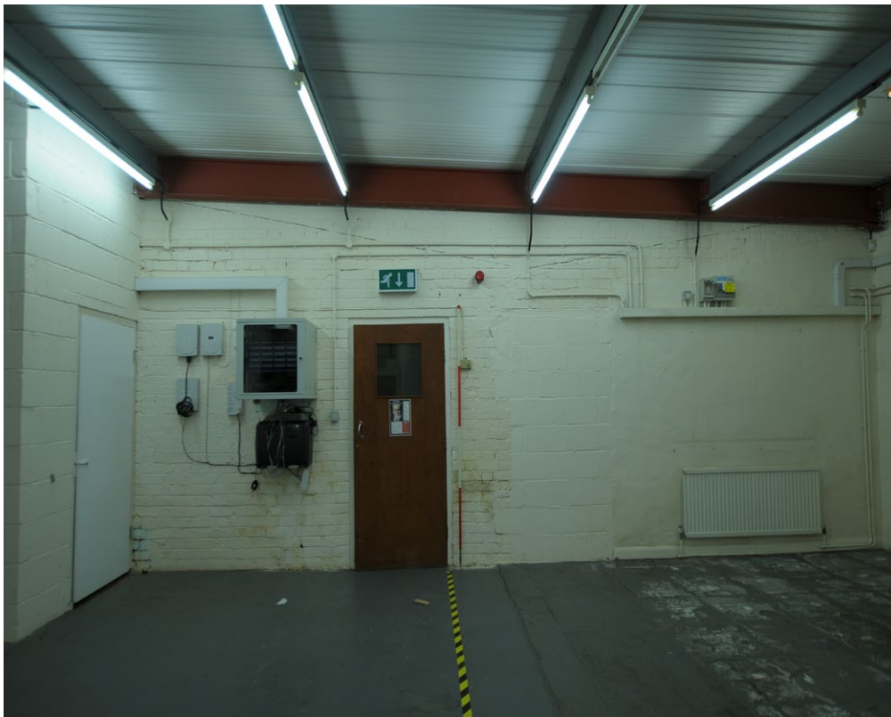
Fig. 9r - The W wall of Unit 3 showing the original 19th century roof line, facing W
