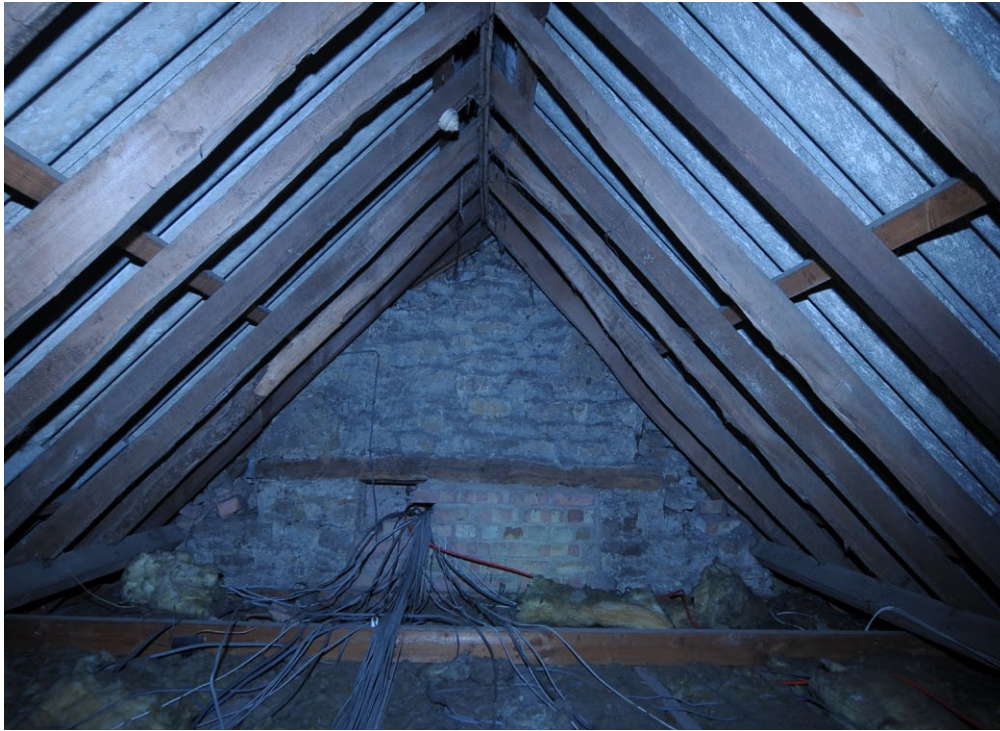
Fig. 9e - Blocked window in west gable of Unit 1, facing W
