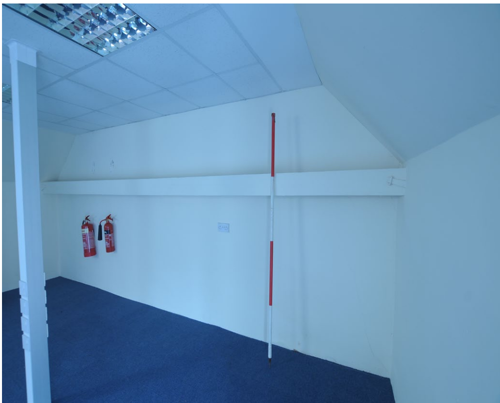
Fig. 9j - The low tie beam on of the E truss, Unit 1, facing E
