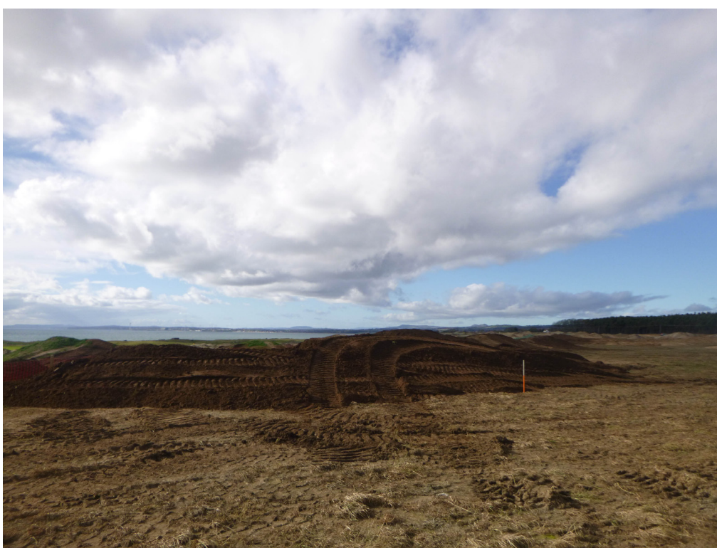
Fig. 3 - General shot of upfilled ridge along the southern extent of the area
