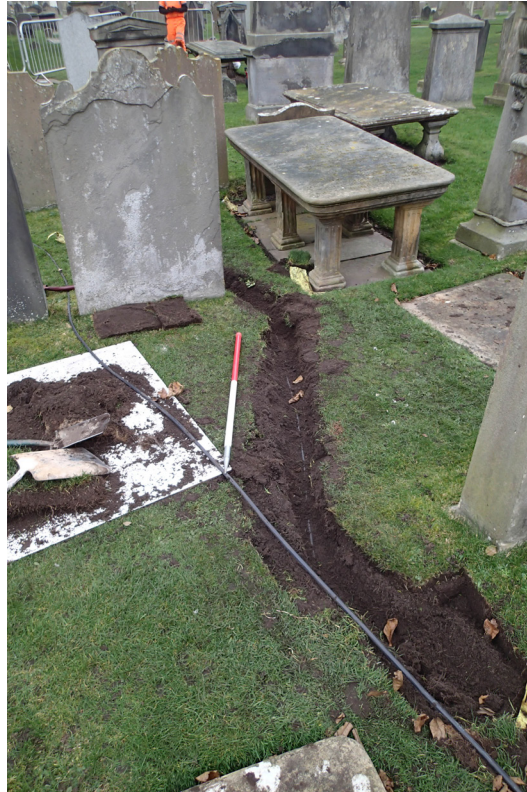
Fig. 6 - General shot showing cable trench weaving between graves at SE corner of St Rules Tower
