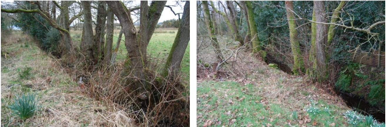
Illus 43 L: line of alders below the drain culvert (PQ C98) R: main drain runs west along the cottage garden edge (PQ C103)
