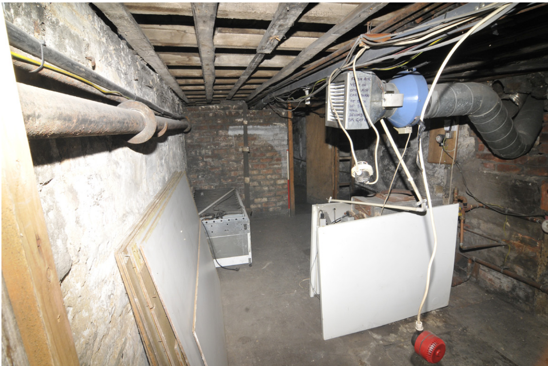
Fig. 17 - Boiler room with services
