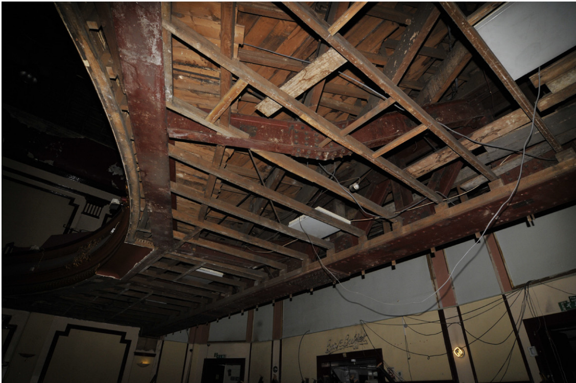
Fig. 15 - Underside of the first floor balcony with cladding removed exposing a Pratt truss spanning the width of the auditorium with bolted raker girders and original 19th century wooden form work
