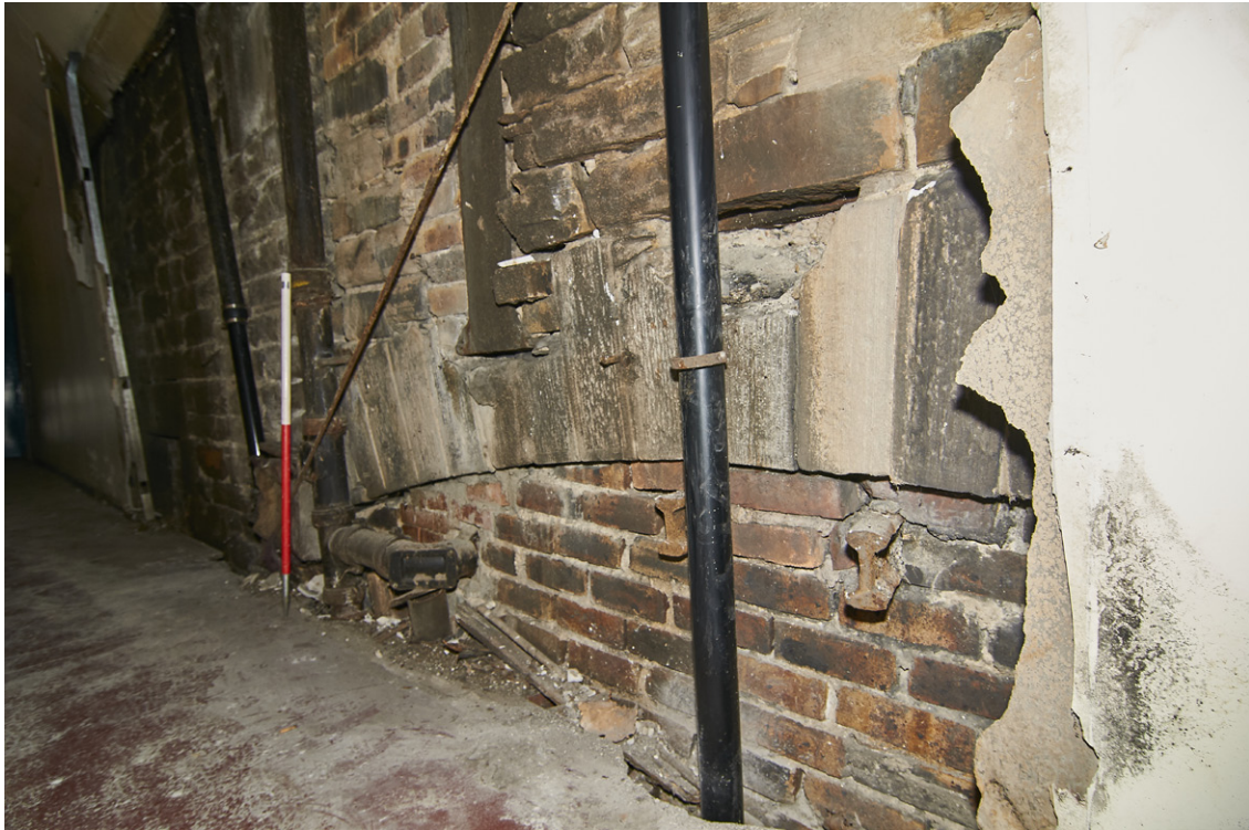
Fig. 6 - Unit 2.1, historic fabric exposed where the cladding had been removed in incorporating a relieving arch blocked with brick and two sections of railway line
