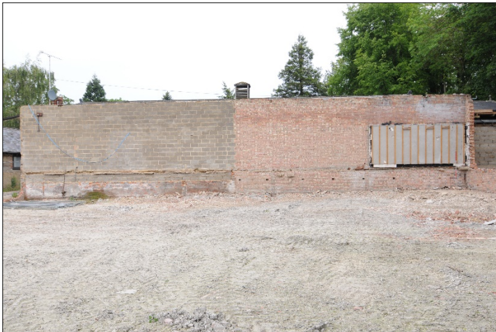
Photograph 7: Breeze block and brick construction of demolished shed forming south-west elevation of stable block
