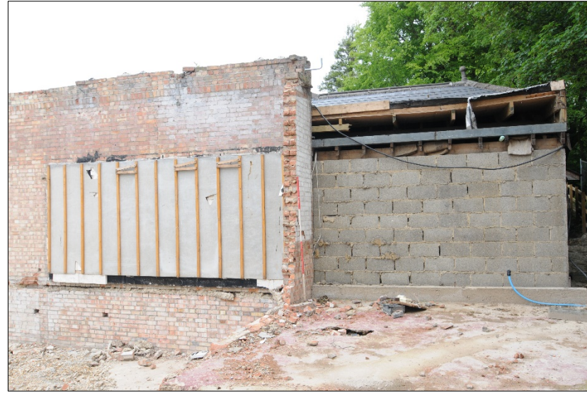
Photograph 6: South-west elevation of stable block showing brick wall of demolished shed and south-east end of stable block
