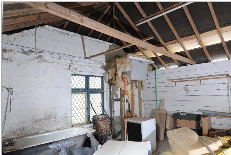
Photograph 23: Interior view of Room 9 at south-east end of stables showing a water tank
