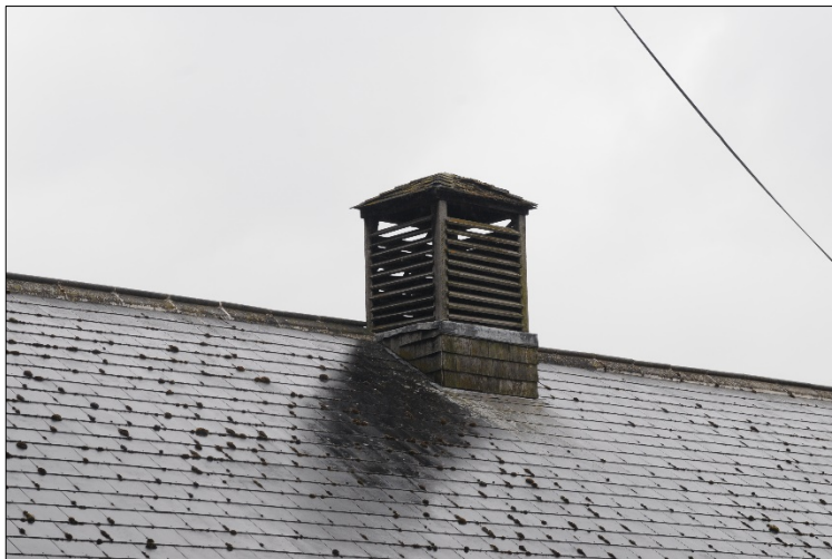
Photograph 19: Wooden ventilator hood on the north east pitch of the stable roof
