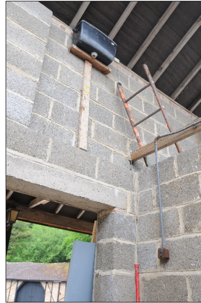
Photograph 28: Cistern to control water flow to the drinkers in each stable
